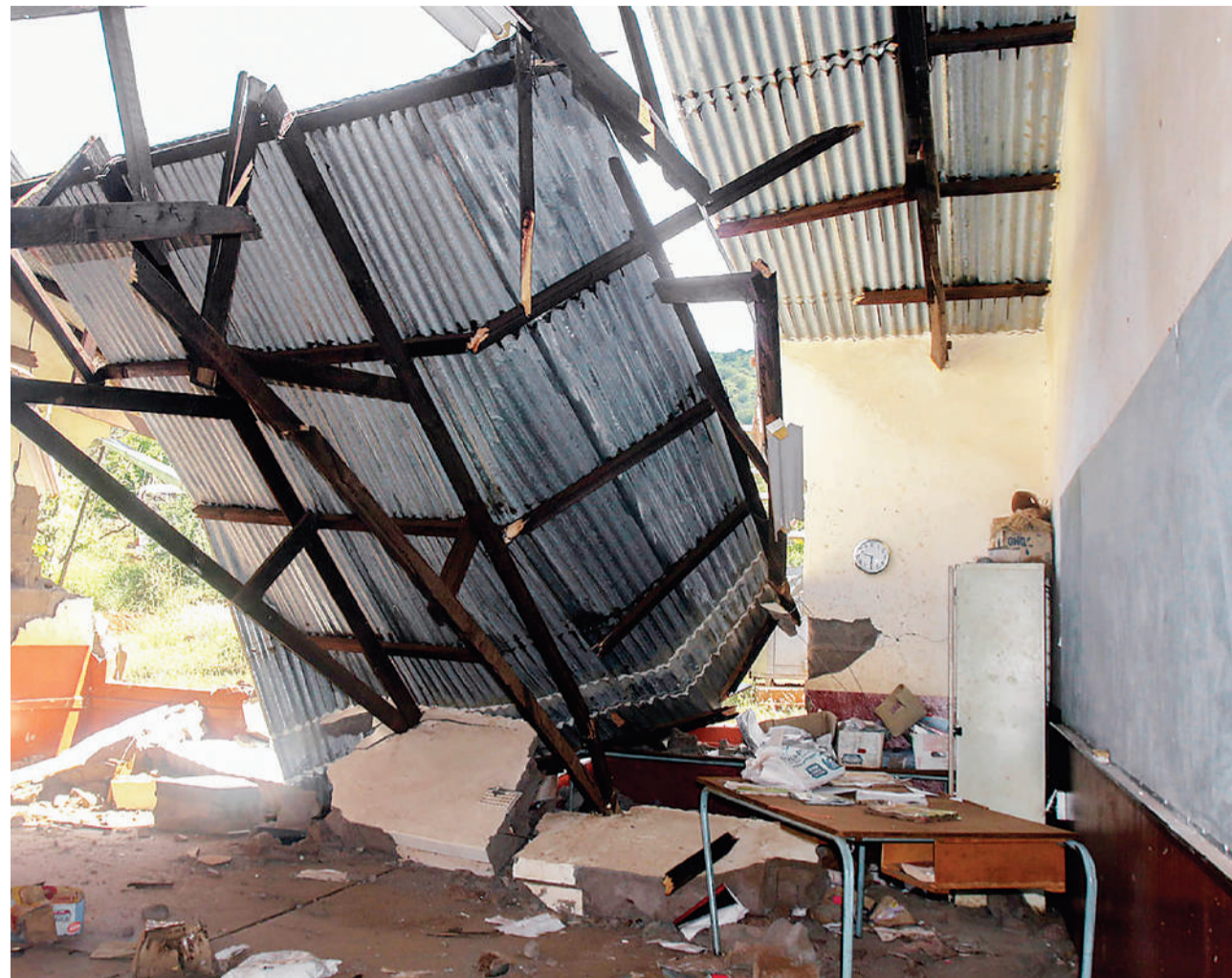
A destroyed roof at Mohloping Primary School in Motlouela village near Burgersfort in Limpopo on 17 January 2018. (File photo)
