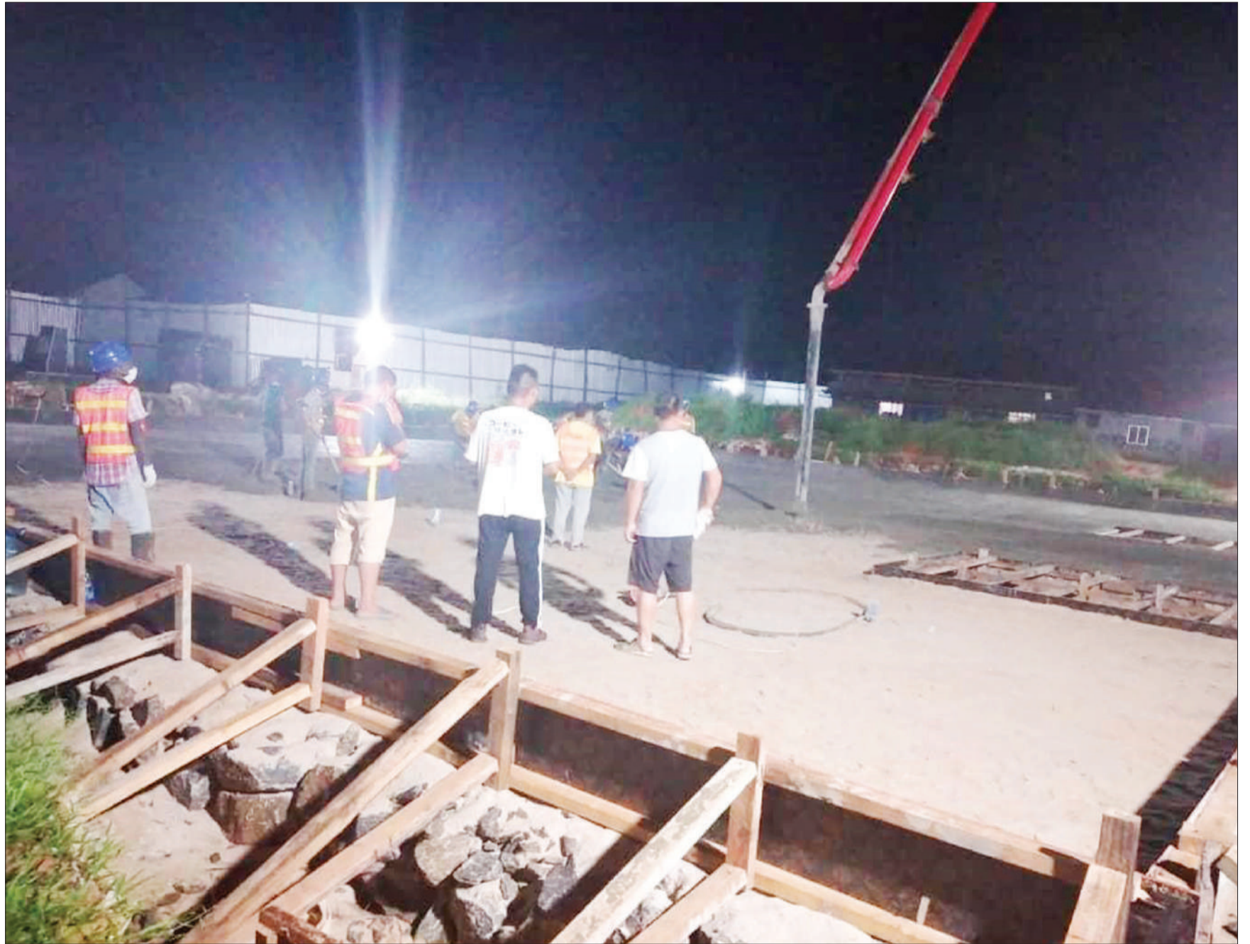
Preparations for the installation of a 2-million-litre water tank under the Kisarawe-Pugu project have begun at Pugu Kajiungeni in suburban Dar es Salaam. The project, which is being implemented by the Dar es Salaam Water and Sanitation Authority (Dawasa), is meant to supply potable water to Kisarawe District in Coast Region as well as Dar es Salaam's Pugu, Gongo la Mboto, Airwing, Ukonga, Kigogo and Majohe suburbs. Photo: Guardian Correspondent
