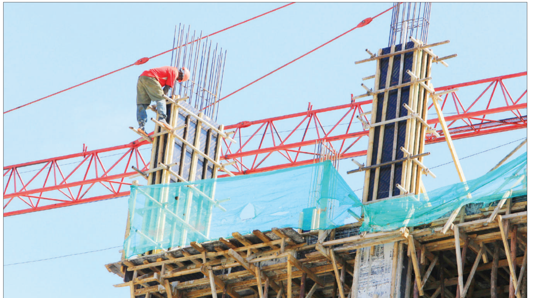
A mason at work on the sixth floor of an investment building in Dodoma, as captured yesterday. There has been a noticeable rise in the number of such complexes in the city since more and more government activities shifted to the new national capital. Photo: Correspondent Ibrahim Joseph
