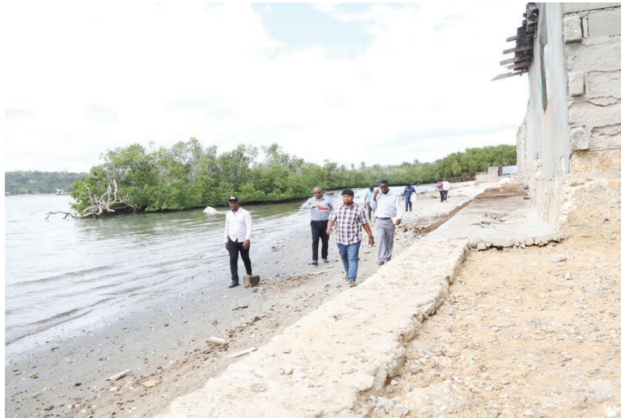
Deputy Permanent in the Vice President's Office (Union) Abdallah Mitawi (2nd L) being briefed on the proposed construction of walls and groynes along Mikindani beach in Mtwara Region yesterday.
