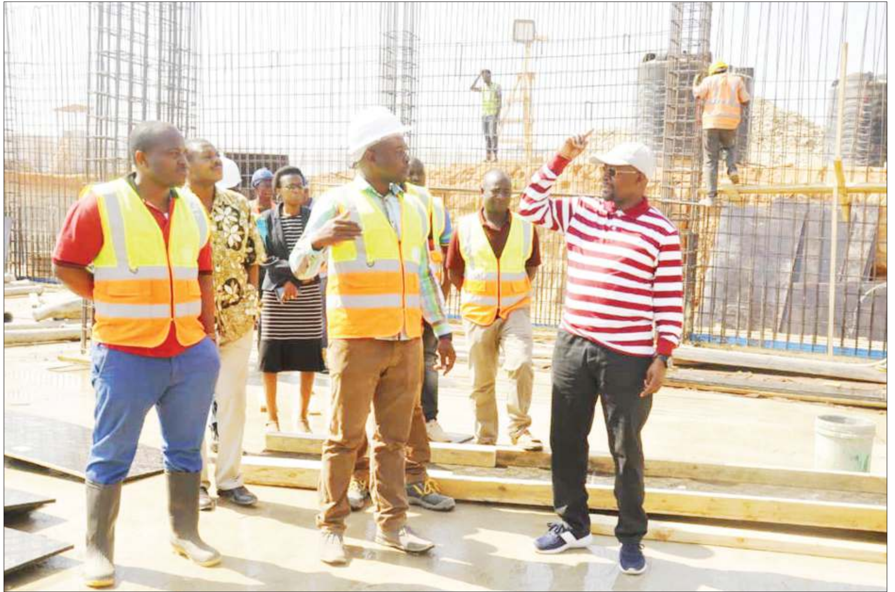
Home Affairs ministry deputy permanent secretary Ramadhani Kailima (R) makes a point at the weekend while on an inspection tour at the site where the Immigration Department headquarters building is under construction in Dodoma city. Photo: Home Affairs ministry
