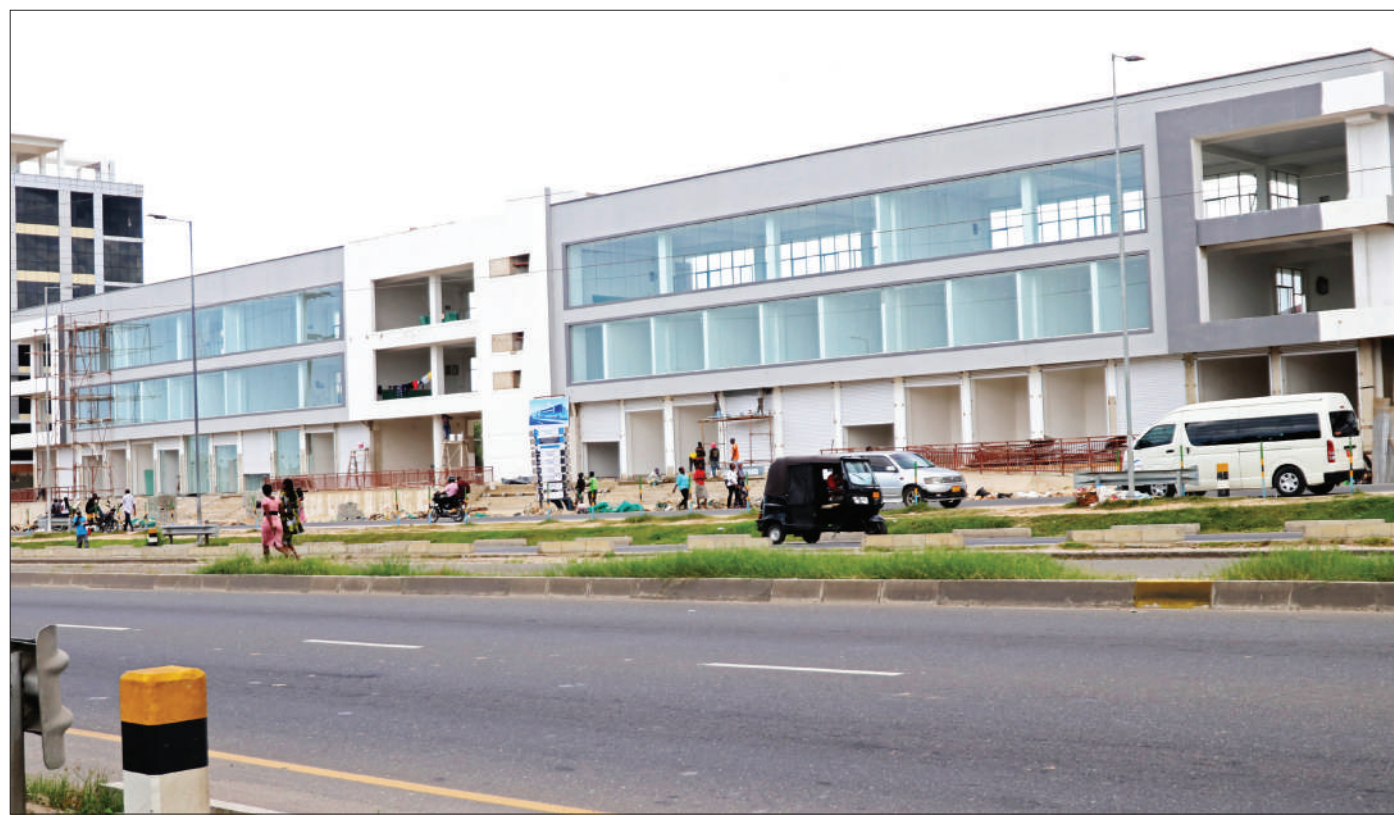
This is how what Kinondoni municipal authorities are developing in Dar es Salaam's Mtwara suburb into a modern commuter bus station currently looks, complete with structures to accommodate shops and various other facilities. The scene was captured yesterday afternoon. Photo: Guardian Photographer
