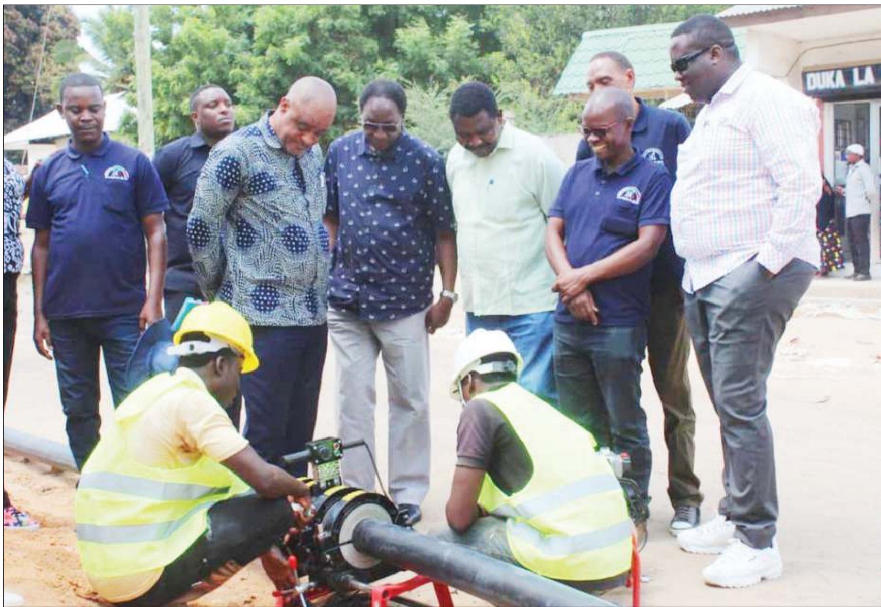
Dar es Salaam Water and Sewerage Authority (Dawasa) board chairman General (retired) Davis Mwamunyanze (C, in eyeglasses) with some members of the board during an inspection tour of the agency's infrastructure in Mkuranga District, Coast Region, yesterday. Photo: Guardian Correspondent
