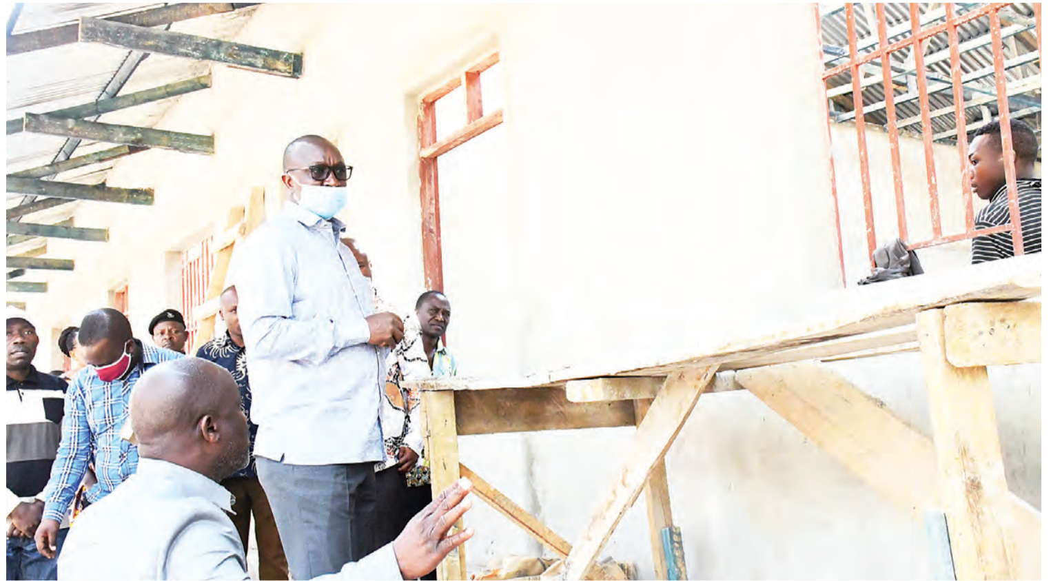
Shinyanga regional commissioner Dr Philemon Sengati (in mask, sun glasses) on an inspection tour of ongoing construction of classrooms at the region's Bugomba B Primary School yesterday. Photo: Correspondent Anthony Ishengoma
