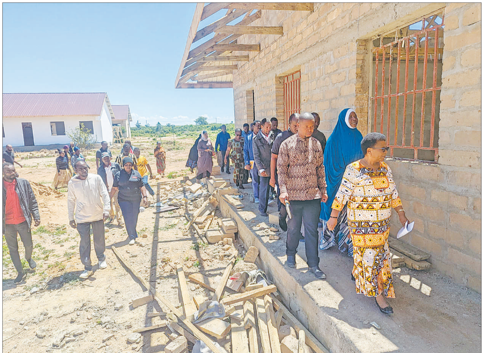
Singida Regional Administrative Secretary Dr Fatuma Mganga (R), inspects construction of a new secondary school at Kintandaa Village, Mtunduru Ward in Ikungi District at the weekend. The school will feature eight classrooms, two teachers' offices, administration block, laboratory, ICT room, water tank, incinerator, toilets stalls and furniture. Photo: Correspondent Thobias Mwanakatwe
