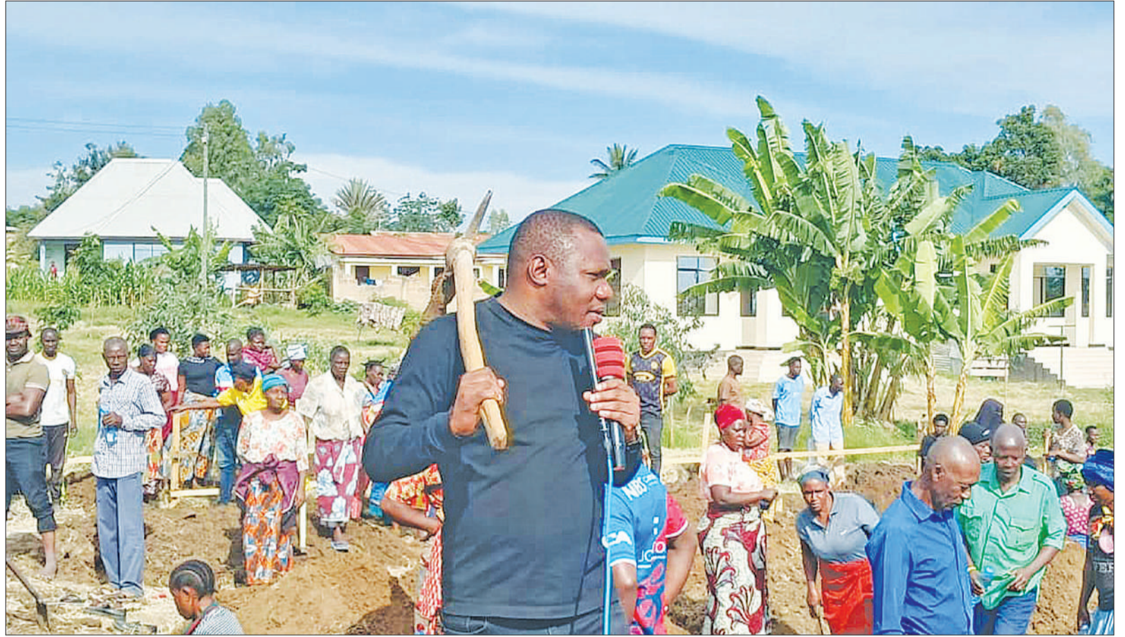
Musoma District Commissioner Juma Chikoka speaks to residents of Kigera Etuma Village before participating in digging of a foundation for the construction of Kigera Mwiyaale Secondary School at the weekend. Photo: Correspondent
