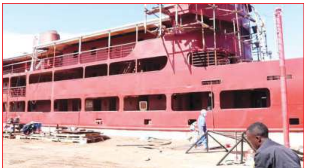
Rehabilitation of MV.Victoria in progress at Mwanza South Port. The Project is implemented by KTMI Co. Ltd from South Korea in Joint Venture with Yuko's Enterprises (EA) from Tanzania and is expected to be ready by March, 2020. This project is implemented concurrently with the rehabilitation of MV.Butima by the same contractors.
