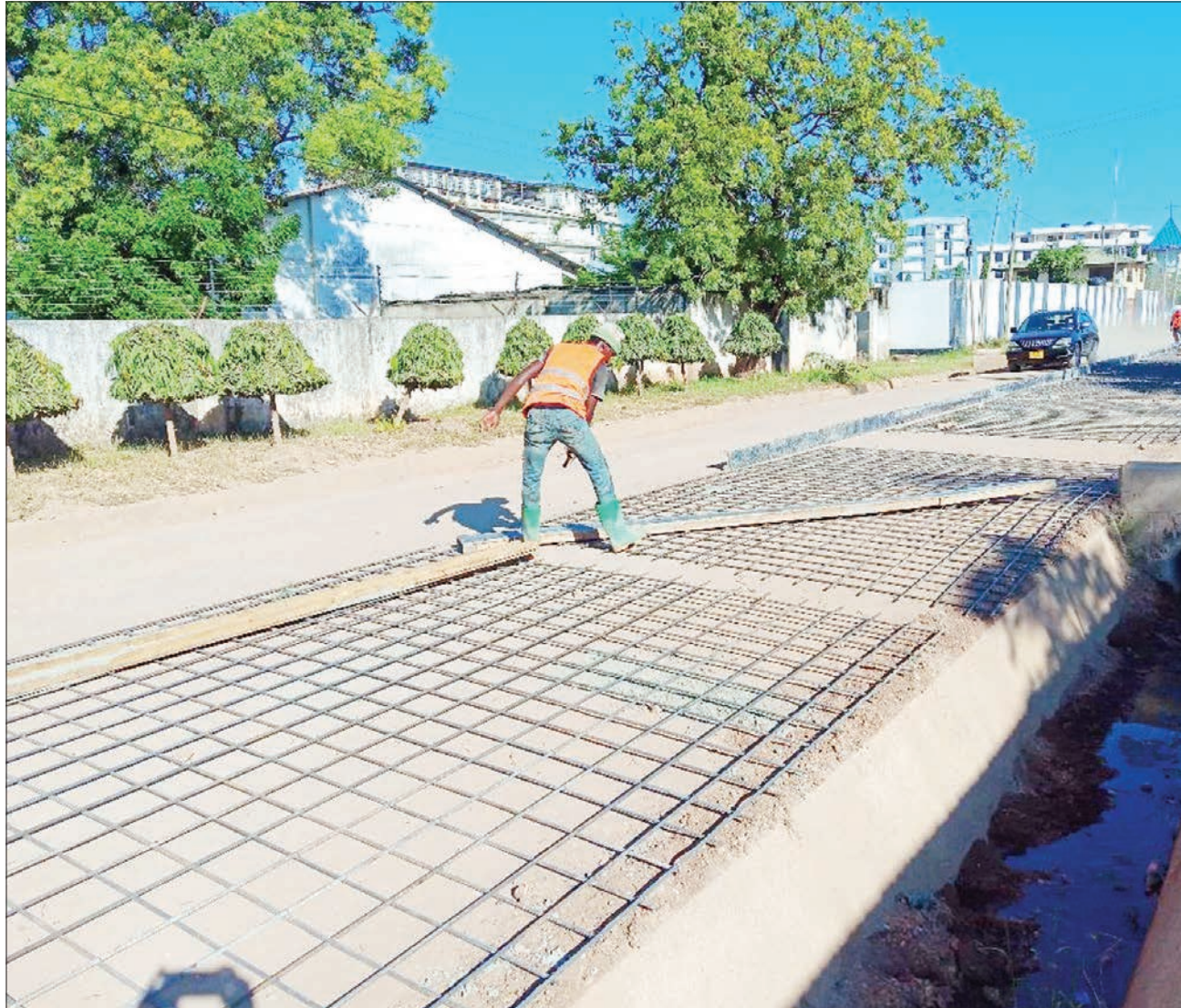
Sewa Road, which traverses Dar es Salaam's Mikocheni Light Industrial Area and has for years been so 'forgotten' as to become notoriously potholed, is now undergoing rehabilitation in earnest. Correspondent Joseph Mwendapole captured this scene yesterday, but it was not immediately established as to who was behind the idea.
