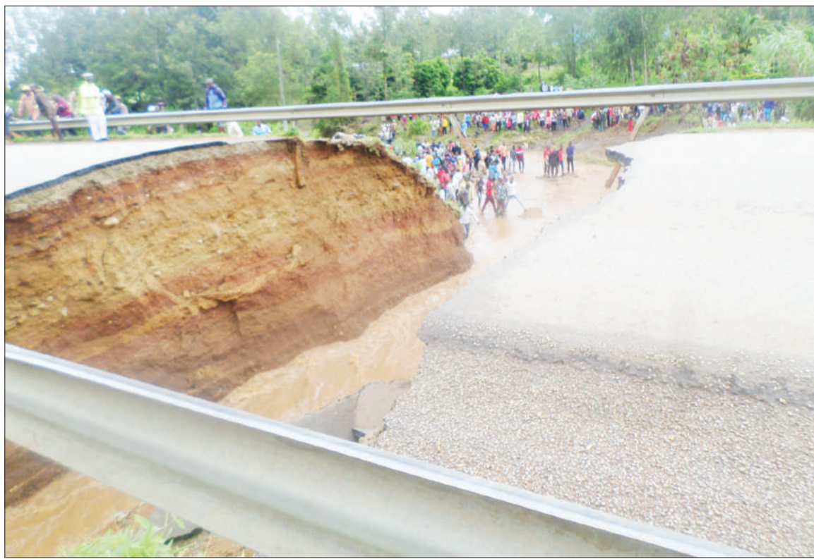
A section of the highway running from Sirari on the Tanzania-Kenya border to Bunda and onwards to Mwanza city has been rendered impassable after floodwaters swept away this bridge at Nyamisangura in Tarime District at the weekend, as captured by Correspondent Samson Chacha
