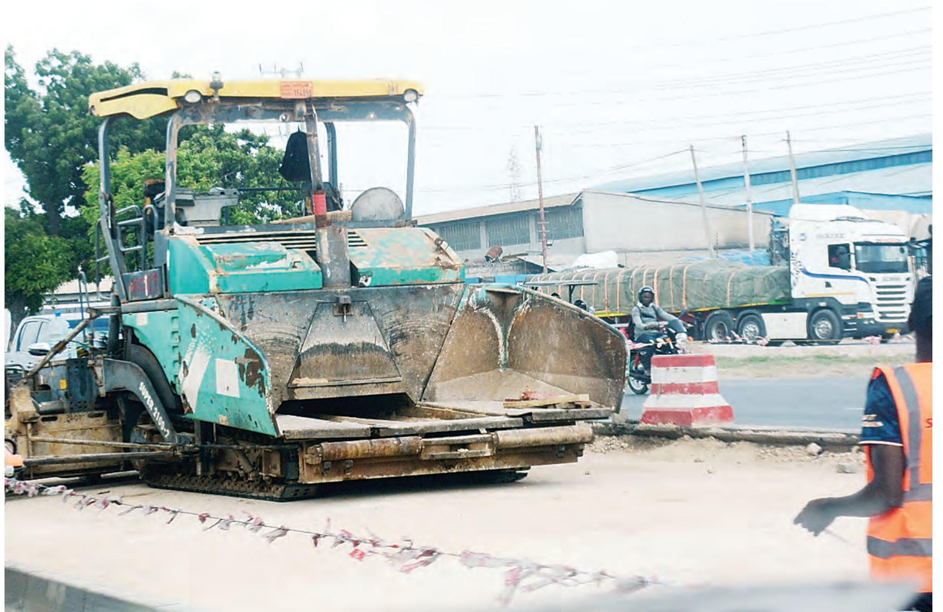
Construction of Bus Rapid Transit (BRT) transport infrastructure well under way in Dar es Salaam's Vingunguti suburb earlier this week. Photo: Correspondent Jumanne
