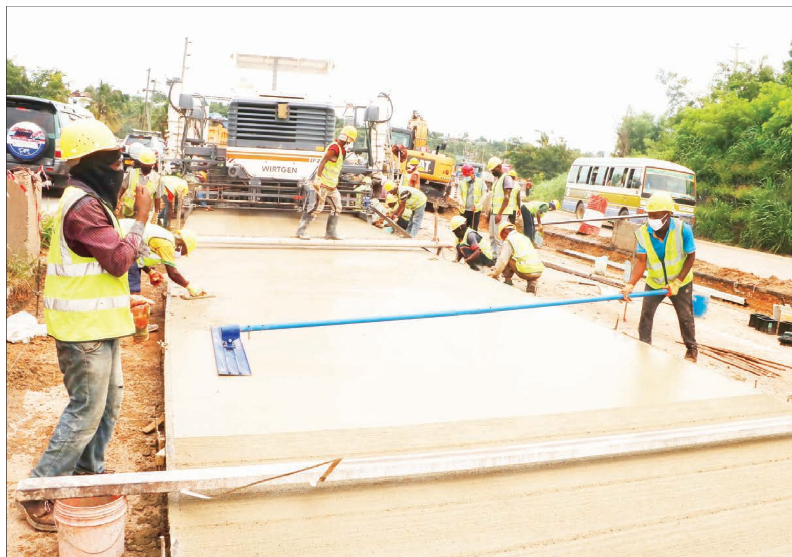
Highway Botek Co. employees levelling concrete as a section of Kilwa Road is resurfaced in Dar es Salaam yesterday. The Dar es Salaam Rapid Transport (DART) phase two plying the Kariakoo to Mbagala Rangi Tatu route will be using the road. Photo: Correspondent Jumanne Juma
