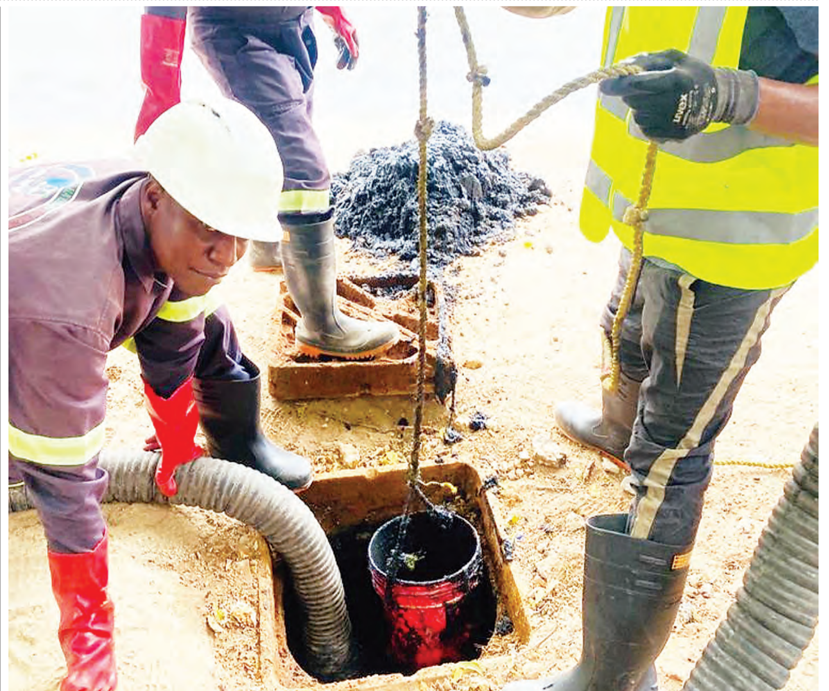
Dar es Salaam Water and Sewerage Authority (Dawasa) technicians clear a clogged sewage system along Ruhinda Street in the city's Upanga-Seaview suburb yesterday. Photo Correspondent Joseph Mwendapole
