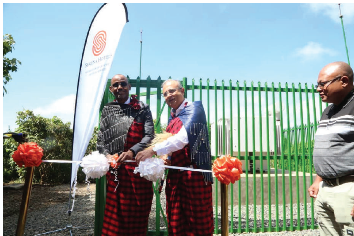
Elirehema Doriye, NCAA Acting Conservation Commissioner (L) shares a word with Ashish Sharma, CEO of Ngorongoro Serena Hotels at the launch of an electricity substation. Looking on is Mbanot Tipilit, Legwainani of the Ngorongoro Maasai community. Photo courtesy of NCAA.
