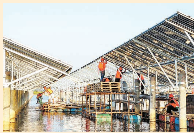
Workers install solar panels at a reservoir in Feidong county, Hefei city, Anhui province. (File photo)
