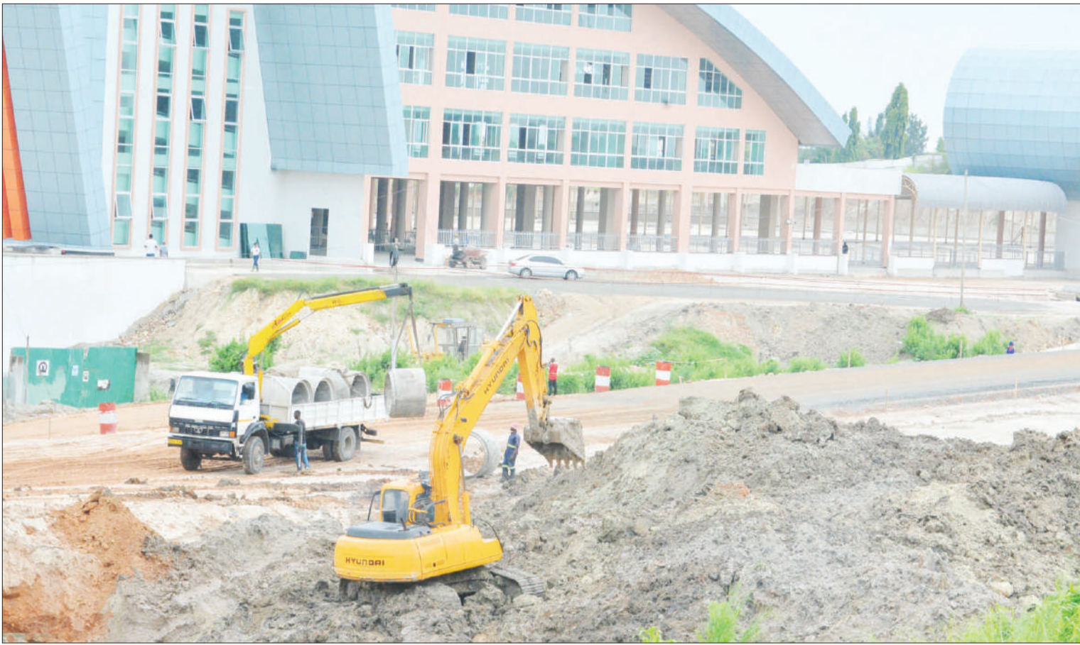
Construction of sewage system in progress at the recently opened modern long-distance bus stand at Mbezi Mwisho in Dar es Salaam, as captured yesterday. Photo: Correspondent Miraji Msala
