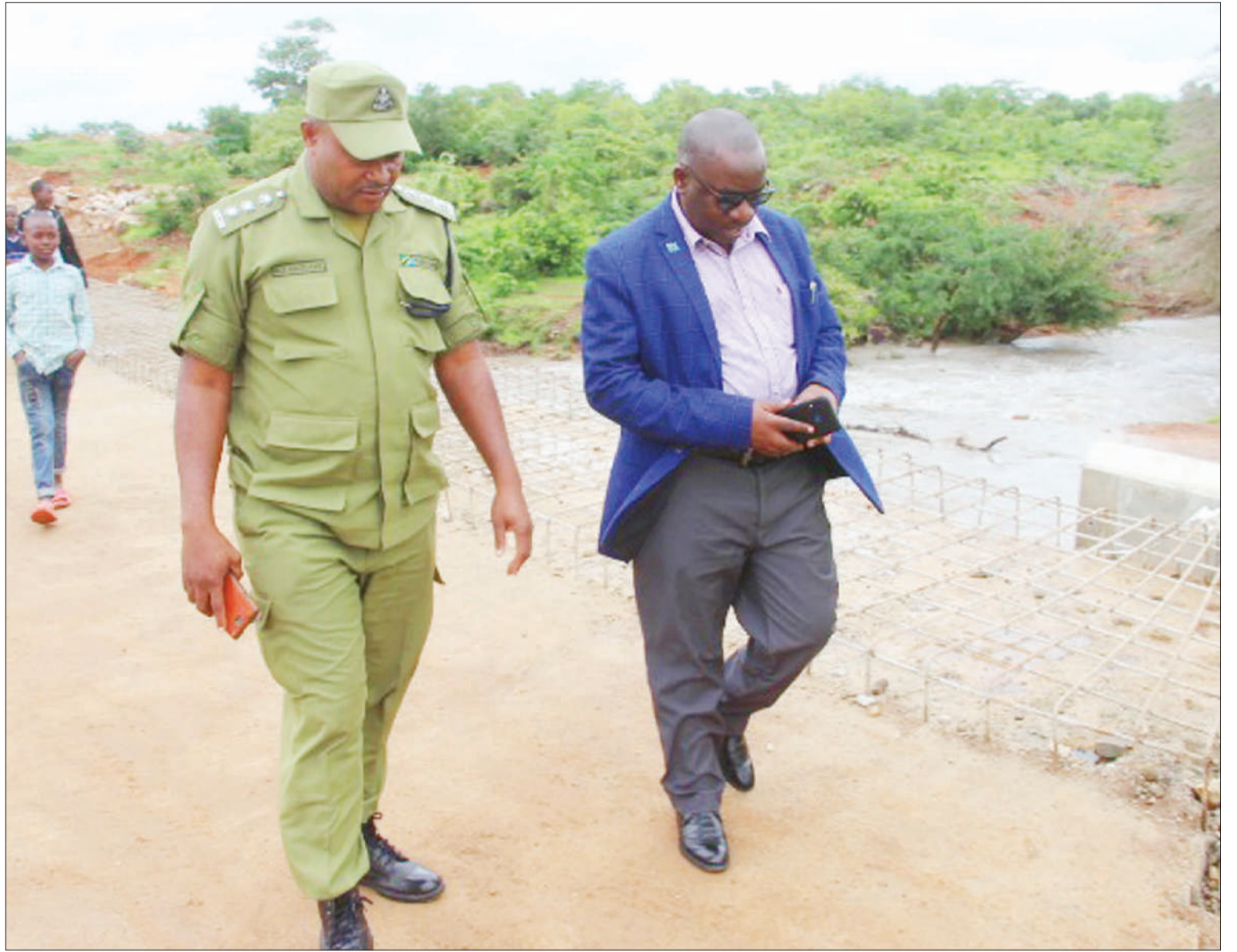
Chunya district commissioner Mayeka Saimon (R) pictured at the weekend assessing progress in the construction of Chunya-Makongolosi bridge. Photo: Correspondent Nebart Msokwa
