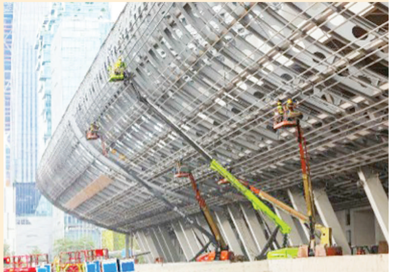
The China Import and Export Fair Complex (Phase IV) is under construction, Sept. 5, 2022. (Photo by Chen Zhiqiang/People's Daily Online)
