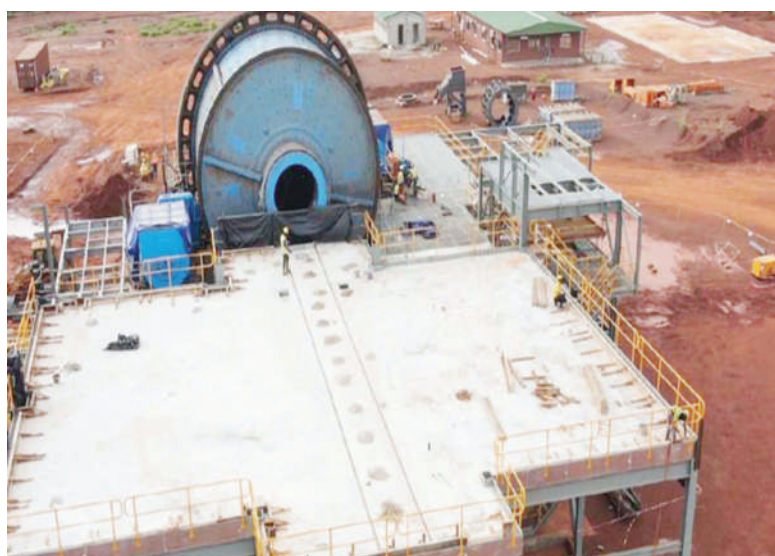
SAG mill construction at Tietto Minerals' Abujar project in Cote d'Ivoire. Credit: File
