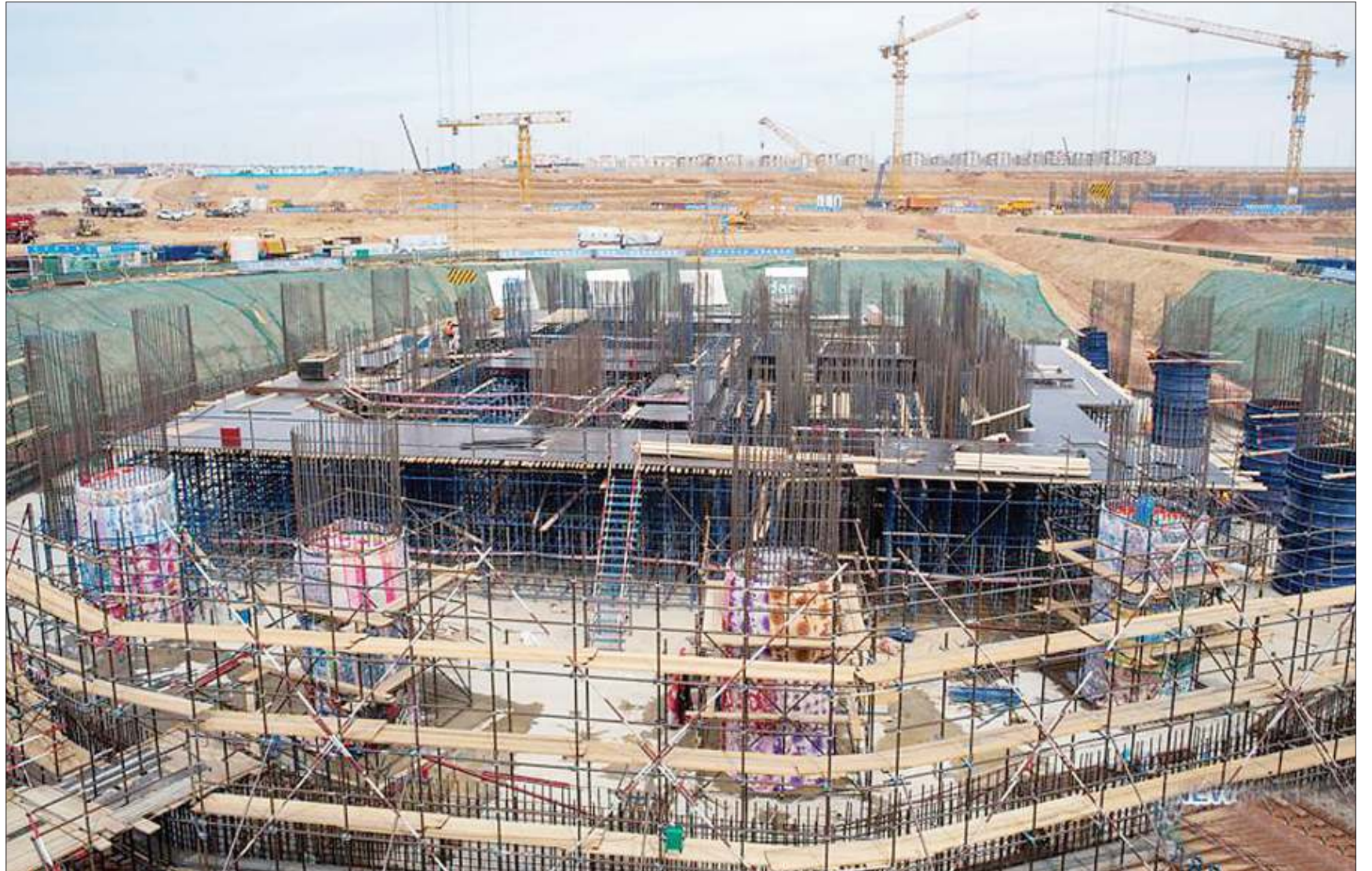
The photo taken on March 12, 2019 shows the construction site of the 385-meter-high Iconic Tower in New Administrative Capital, about 45 km east of Cairo, Egypt. (Xinhua/Wu Huiwo)
