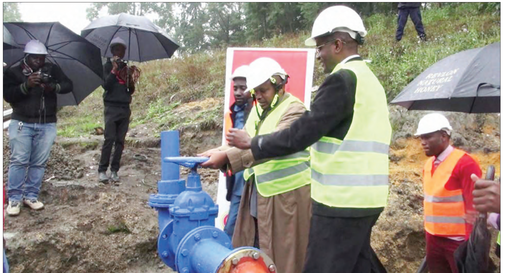
Rungwe district commissioner Dr Vincent Anney opens a pipe at Ikama last week to launch a TOL Gases Limited carbon dioxide plant at the village. Photo: Guardian Correspondent
