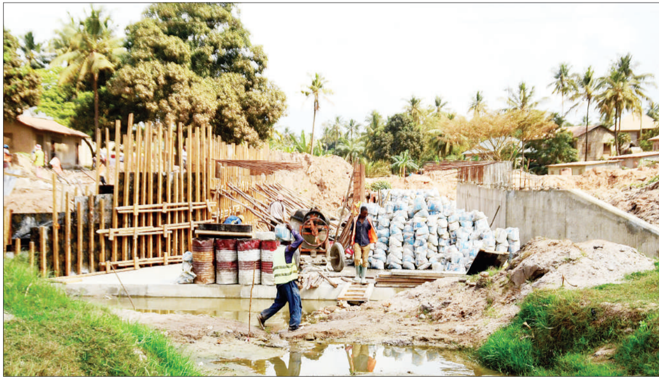
This is a scene Correspondent Jumanne Juma captured yesterday from Kerezange River bridge at Kitunda in suburban Dar es Salaam. It is undergoing construction.
