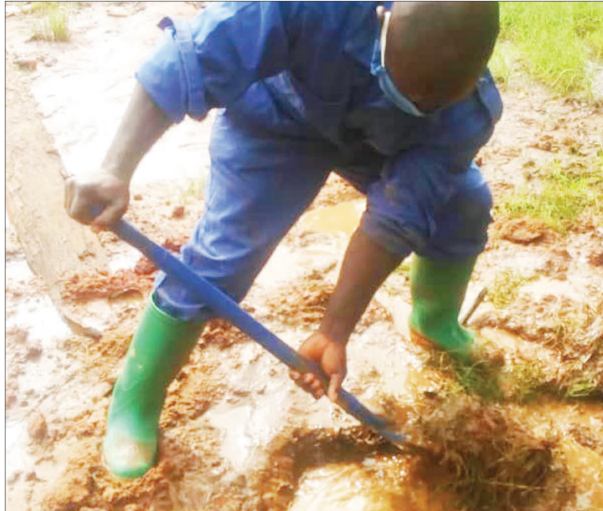
A Dar es Salaam Water and Sanitation Authority (Dawasa) technician moves to replace a leaking pipe at Mlandizi in Coast Region yesterday. Photo: Guardian Correspondent
