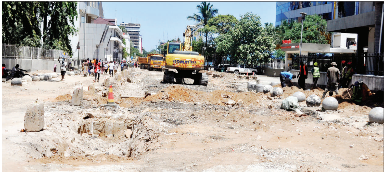
Employees at work to rehabilitate Sokoine Drive in the central business district of Dar es Salaam earlier this week. Photo: Correspondent Imani Nathaniel
