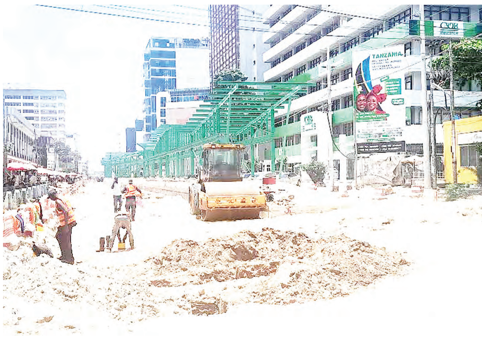
Construction of rapid transit bus stand in progress at New Post Office area in downtown Dar es Salaam, as spotted yesterday. Photo: Correspondent Imani Nathaniel
