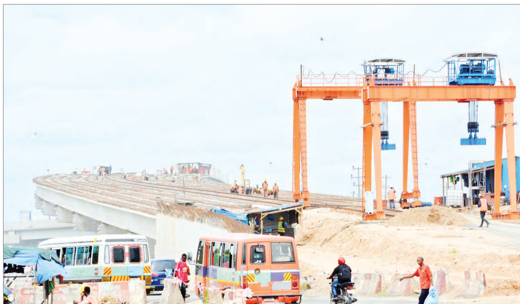
Work on the Ubungo Interchange at the junction of Dar es Salaam's Morogoro, Mandela and Sam Nujoma roads well under way under China Civil Engineering Construction Corporation contractors, as witnessed yesterday by Correspondent Miraji Msala
