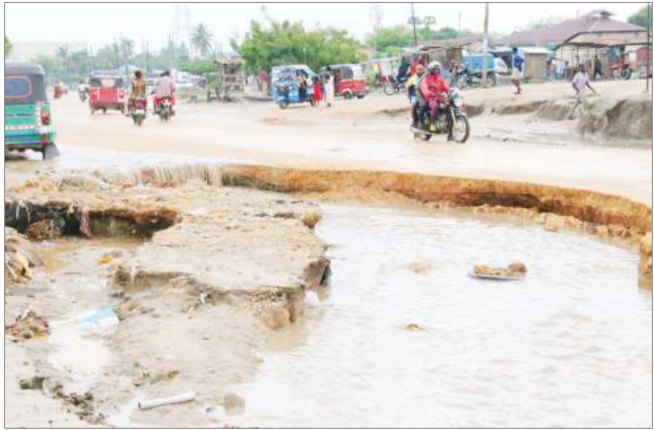
A recently built road in Dar es Salaam's Mbagala Kiburugwa suburb lies badly damaged by the days of heavy rain the city has been experiencing, as captured yesterday. Photo: Selemeni Mpochi
