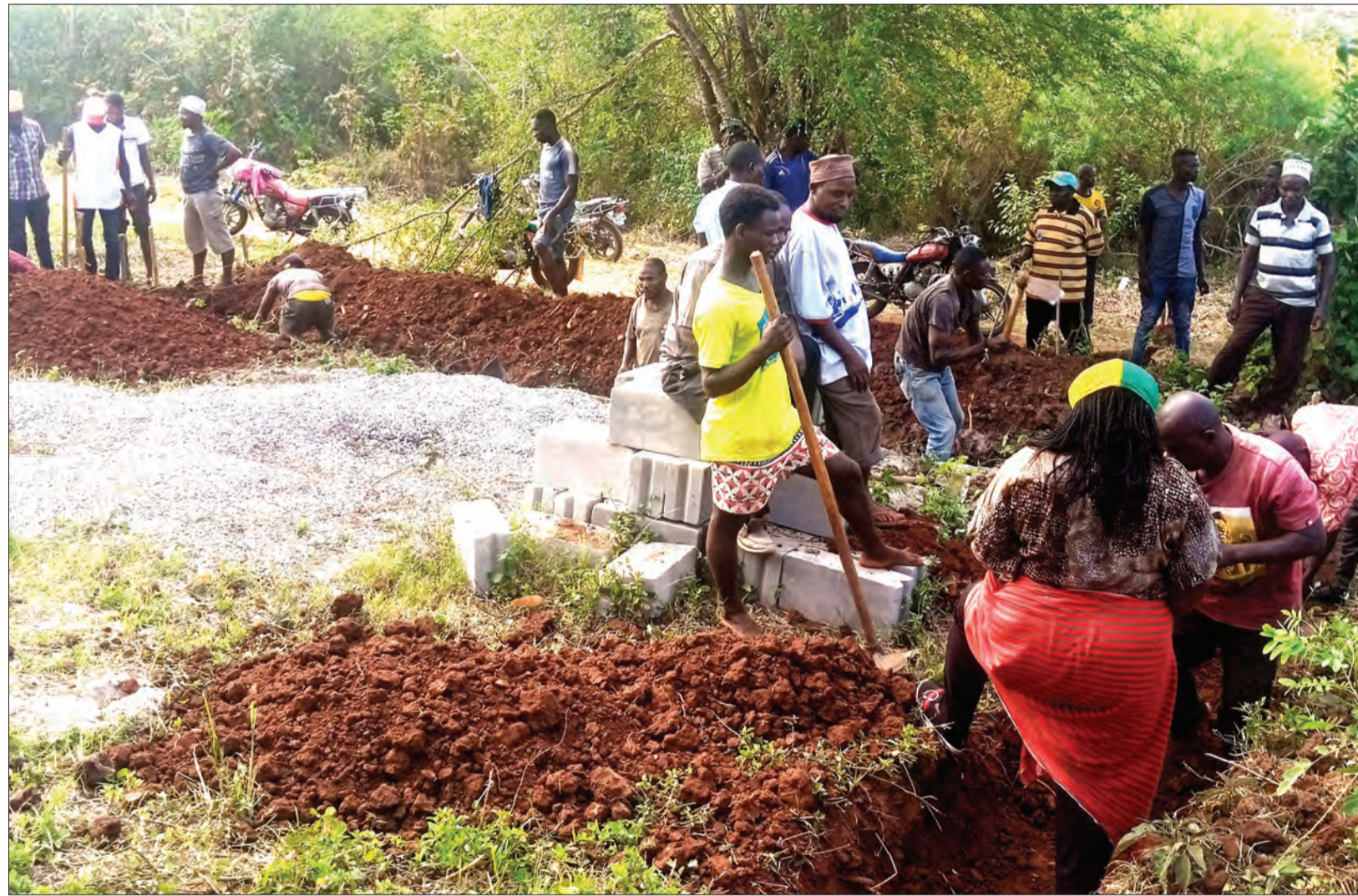
Songwa residents in Muheza district, Tanga region participate in classrooms construction for a secondary school ward recently. Photo: Correspondent Steven William
