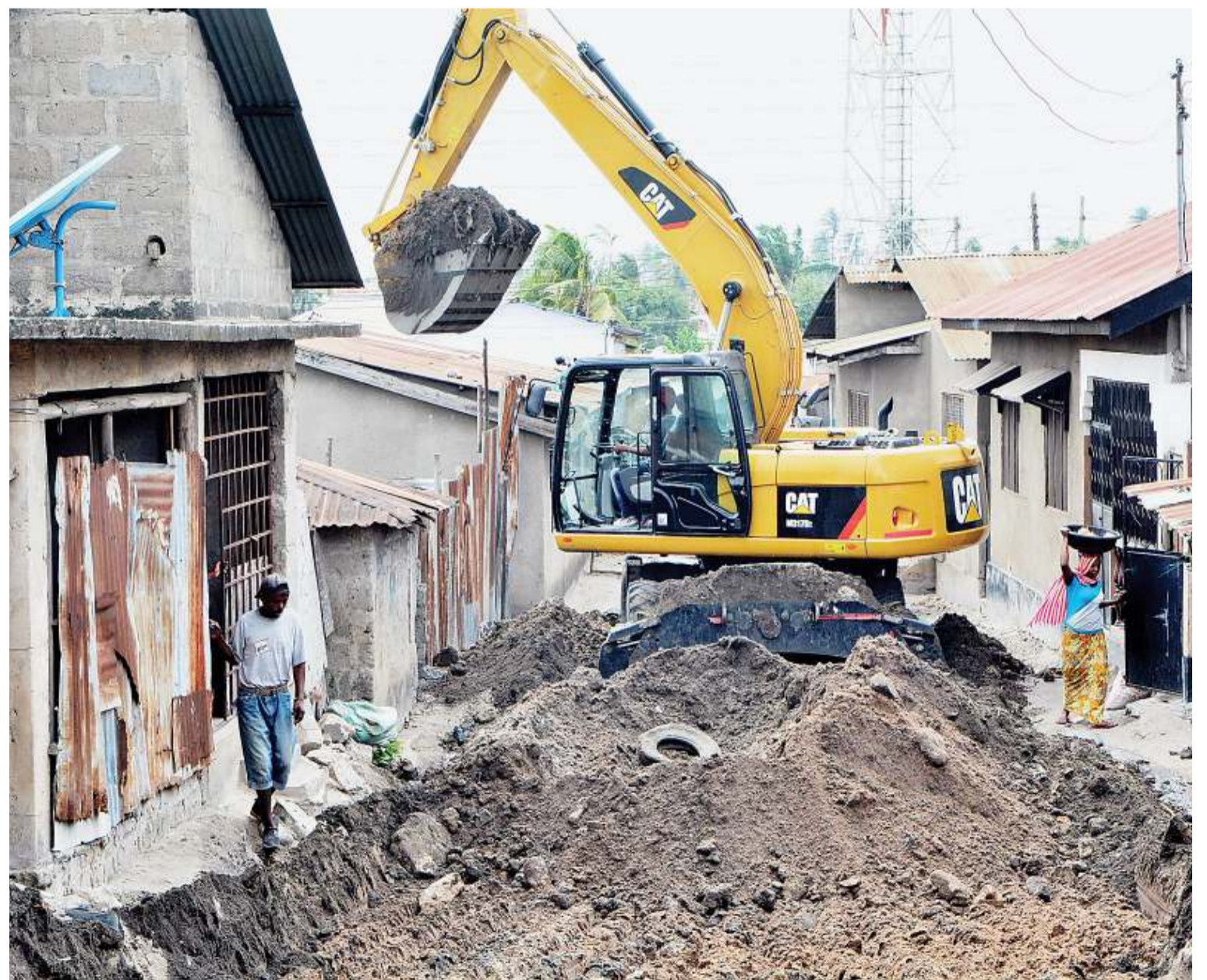
Major works in progress on a road in Dar es Salaam's Tandale kwa Mtogore suburb under the oversight of a Chinese contracting firm, as captured yesterday. Photo: Correspondent Miraji Msala
