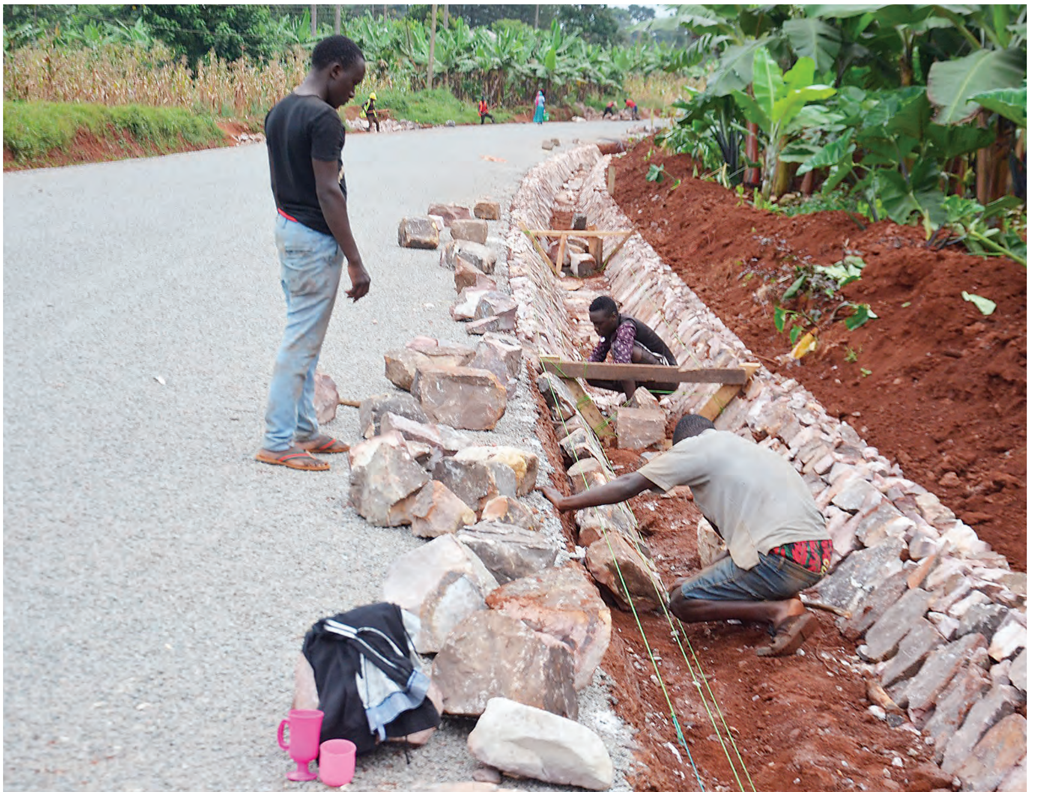
Construction of drainage system in progress on the sides of a trunk road in Muleba District, Kagera Region, late last week. Photo: Correspondent Jumanne Juma
