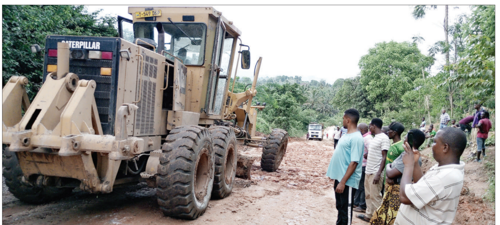
A caterpillar removes mud and debris after heavy rainfall in Matombo division, Morogoro Region yesterday. Passengers' vehicles plying Msamvu-Kisaki were stuck in mud for almost an hour. Photo: Correspondent Christina Mwakangale
