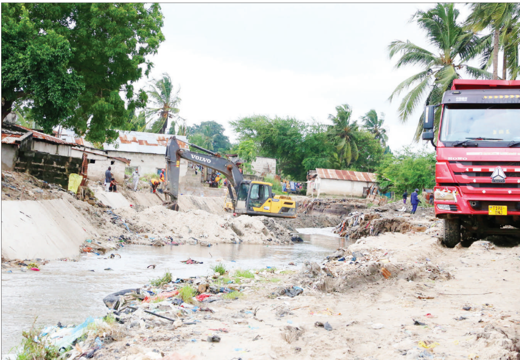
Dar es Salaam's River Ng'ombe undergoes expansion as part of a strategy to spare houses in the neighbourhood the destructive impact of floods. Photo: Selemani Mpochi
