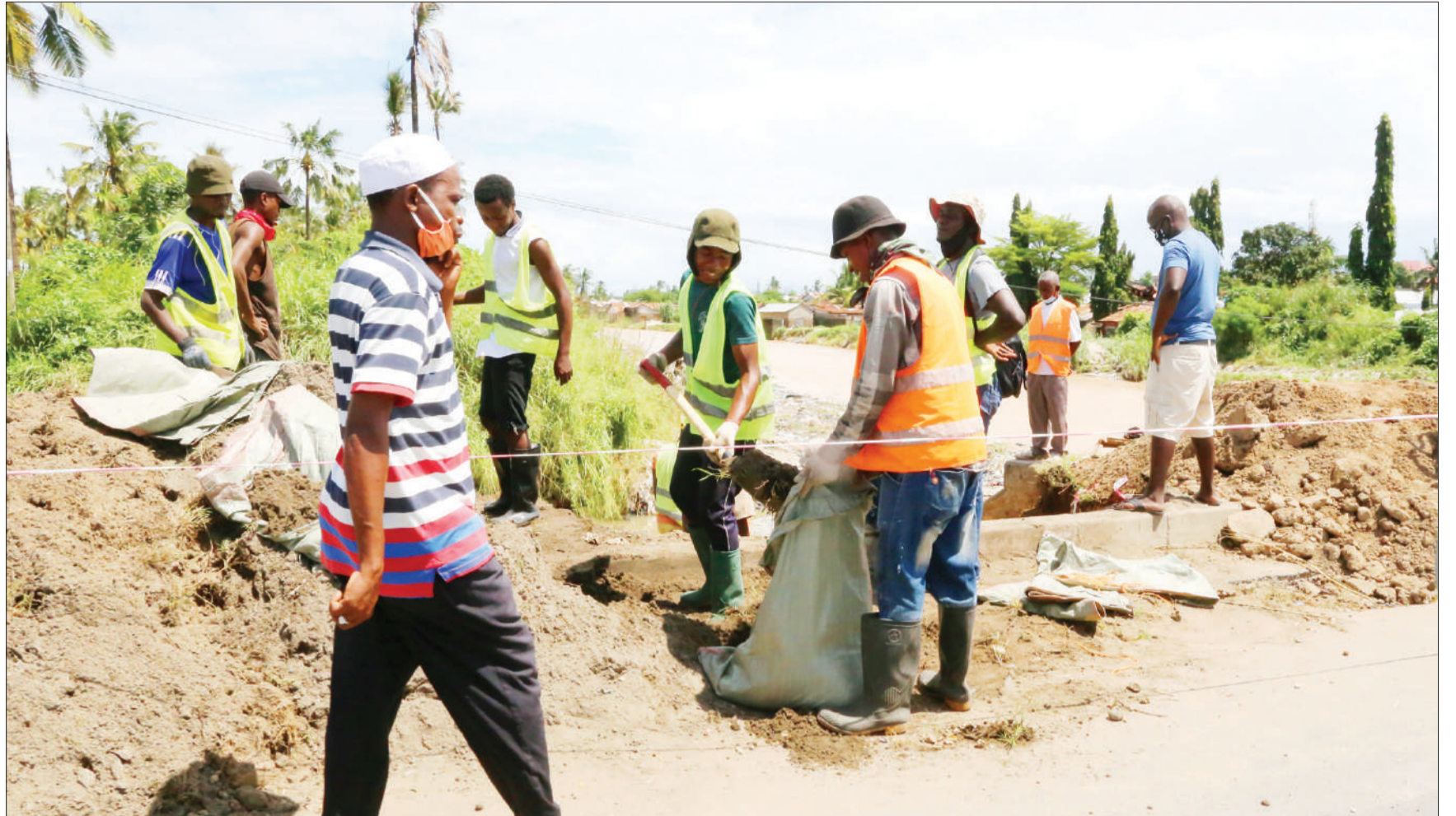
Rehabilitation of a Kigogo Mbuyuni section of a road demolished by floodwaters after the banks of Dar es Salaam's River Msimbazi burst gets under way, as captured yesterday. Photo: Guardian Photographer
