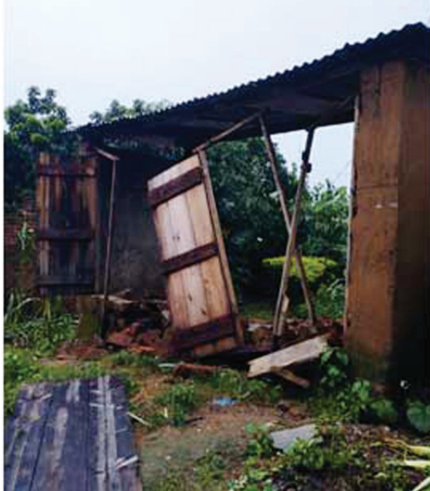
Damage to a road and property in Malawi caused by Cyclone Freddy. Credit: PSGR
