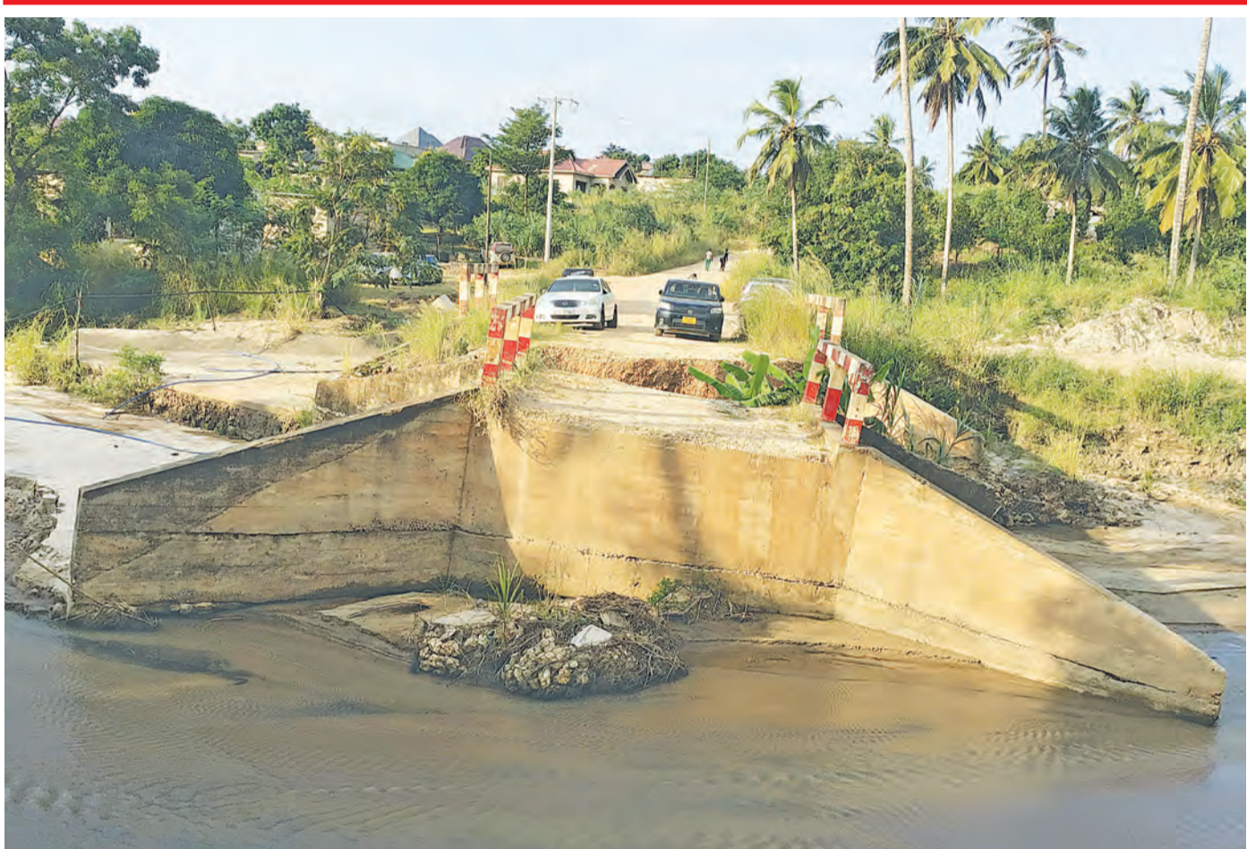
SEVEN MONTHS LATER, BRIDGE STILL KAPUT... It has been all quiet more than half a year since Kwa Ndee Bridge (pictured) fell apart and this section of the road linking Dar es Salaam's Madale Mwisho and Msumi suburbs was rendered impassable. Even the authorities expected - or supposed - to work on the issue or merely comment on it are said to have remained tight-lipped to date. Photo: Guardian Correspondent
