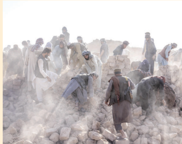
Afghan volunteers clean up rubble after an earthquake in Zenda Jan district in Herat province, western Afghanistan, Oct 11, 2023. (PHOTO/AP)
