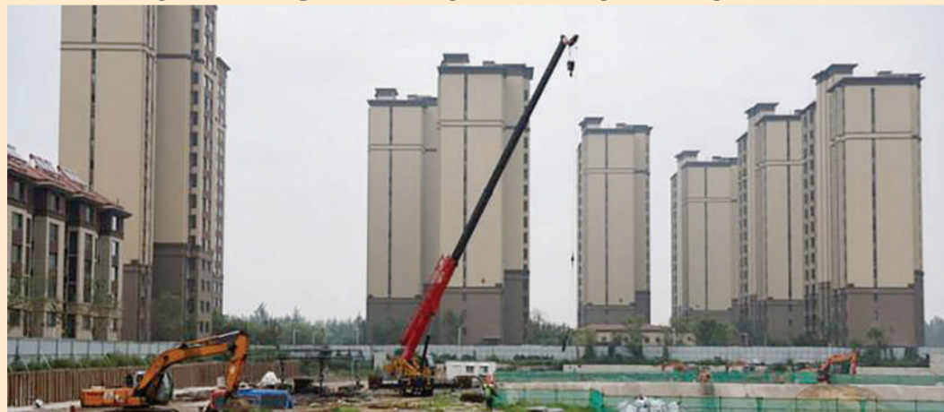
Construction site of residential buildings by Chinese developer Country Garden in Tianjin
