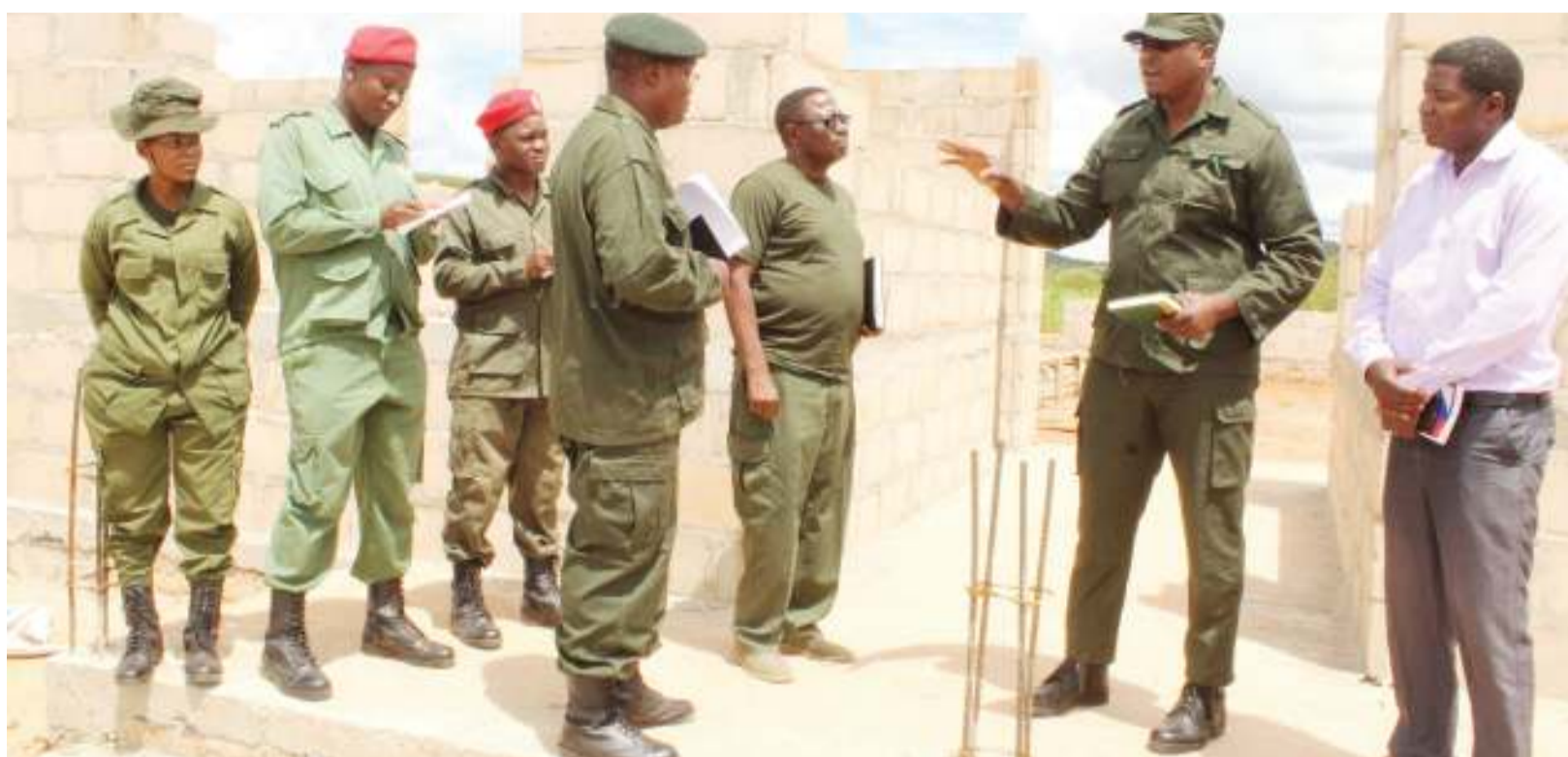
Deputy minister for Natural Resources and Tourism official Constantine Kanyasu gives orders to Swagaswaga Forest manager Alex Choya before the inspection of the ongoing hostel building with the capable to accommodate 77 tourists in Chemba district in Dodoma region over the weekend. Photo: MONT
