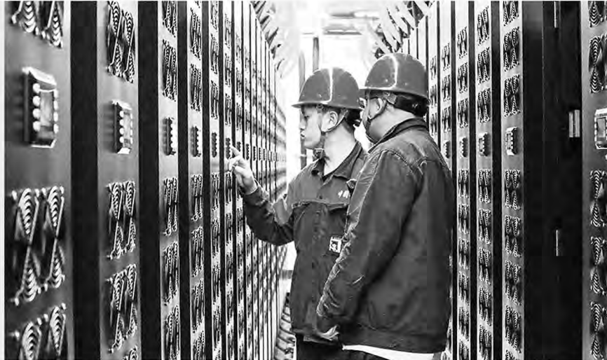
Staff members of the Gui'an Supercomputing Center check the operation of equipment. (Photo by Liu Qing)
