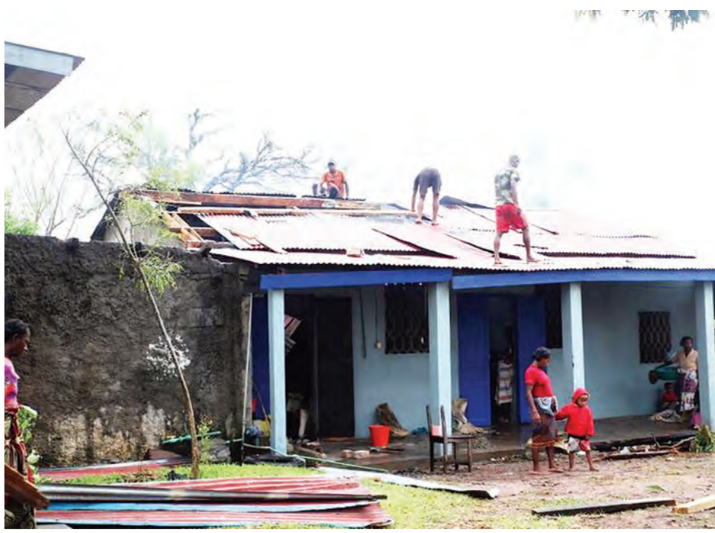
Men repair the roof of a house in the aftermath of cyclone Freddy in Mananjary on Feb 23, 2023. (PHOTO / AFP)
