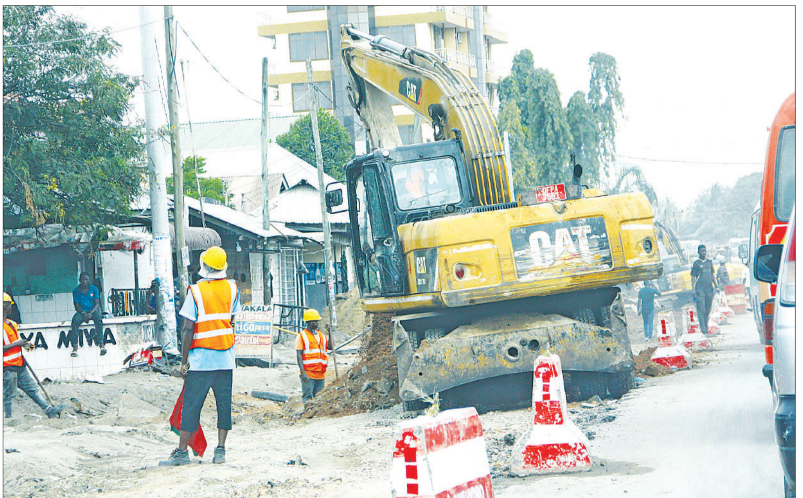
Implementation of Dar es Salaam's rapid transit bus infrastructure project in progress at an Ilala-Bungoni section yesterday. Photo: Correspondent Jumanne Juma
