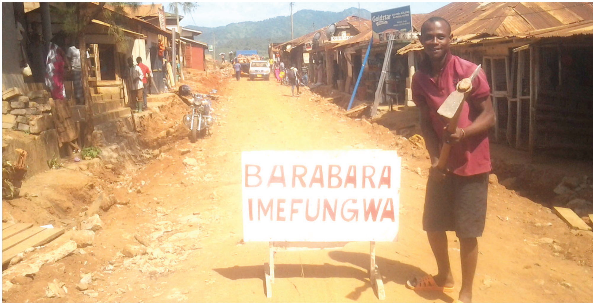
Muheza resident in Tanga region walks next to the road sign which read: The road is closed for rehabilitation yesterday. Photo: Correspondent William Steven
