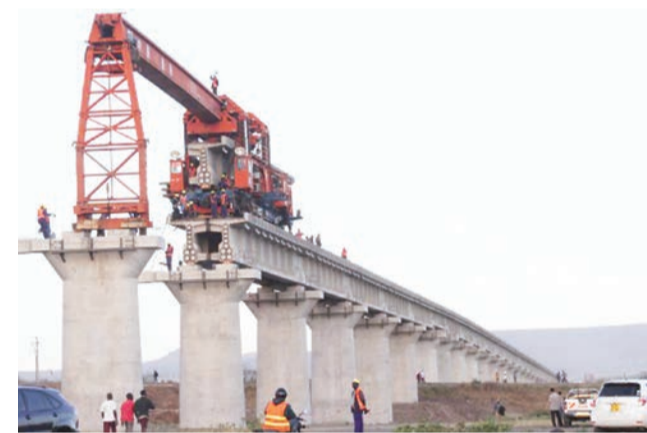
Construction of Standard Gauge Railway currently going has benefitted from CRDB financing.
