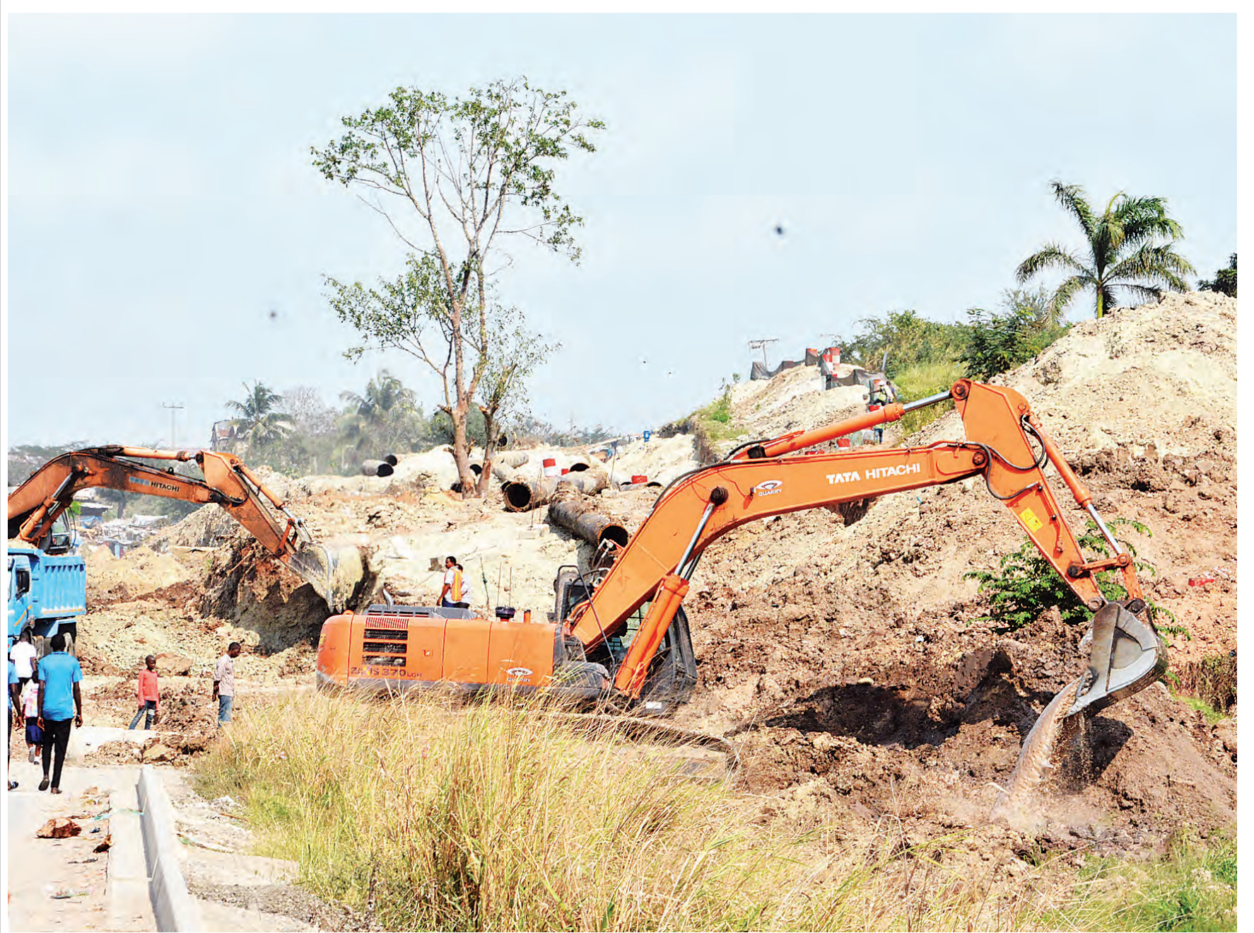
Work under way on the Dar es Salaam Rapid Transit (DART) road infrastructure along the stretch from the city's Mbagala suburb to the city centre, as found at the Uhasibu section of Kilwa Road yesterday. Photo: Correspondent Jumanne Juma
