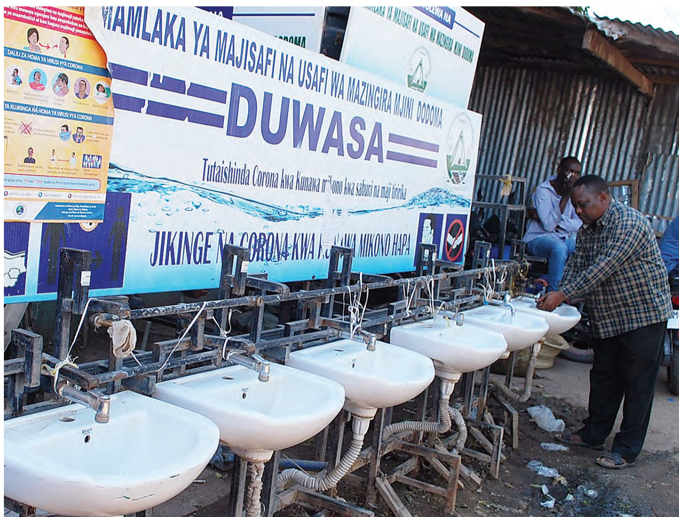
A Dodoma resident washes his hands at the entrance of the city's Majengo main market yesterday, but with most of the taps defective. Photo: Correspondent Peter Mkwavila
