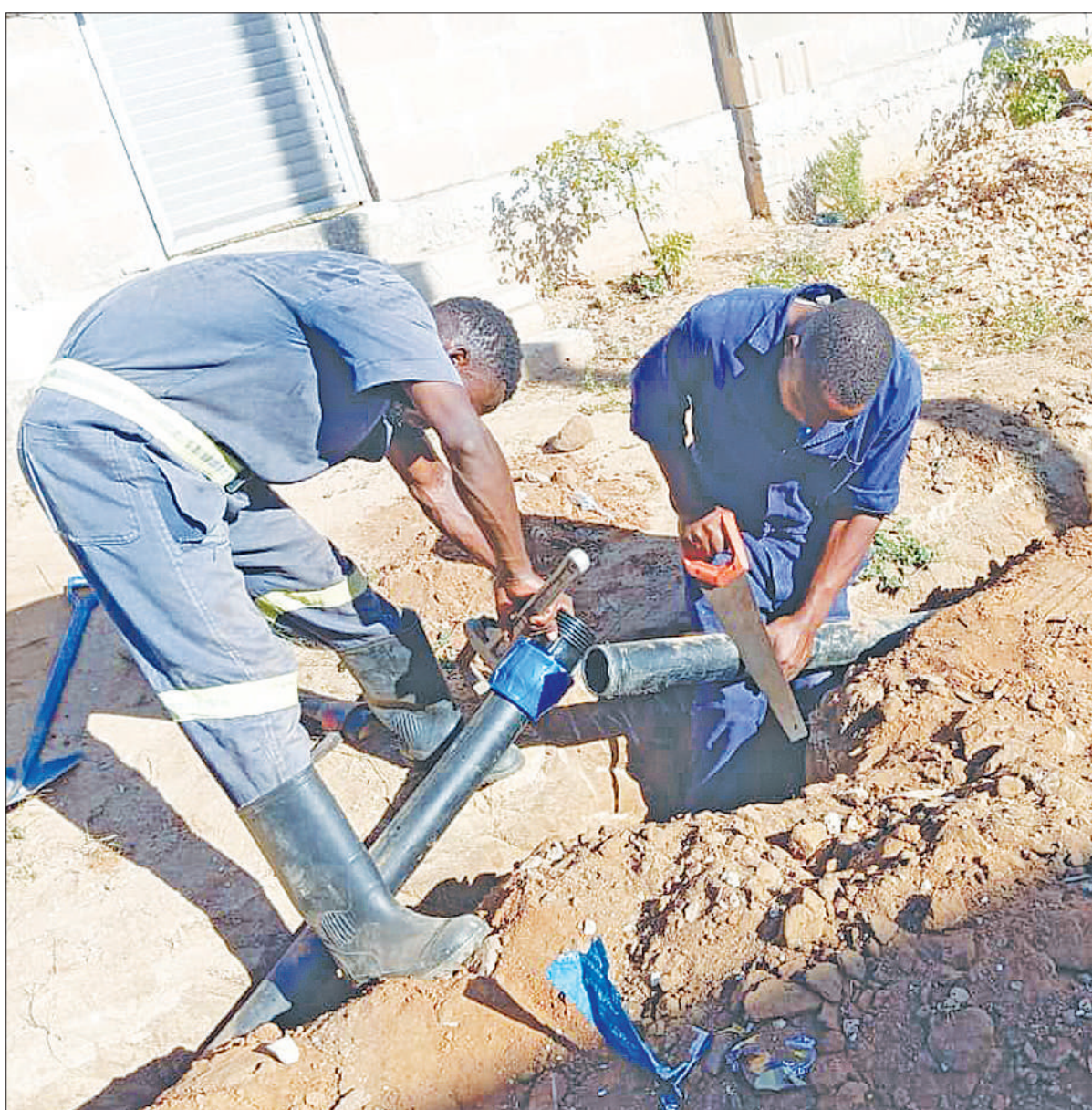
Dar es Salaam Water and Sanitation Authority (Dawasa) technicians connect water for distribution to a section of Dar es Salaam's Tegeta suburb yesterday. Photo Correspondent Joseph Mwendapole
