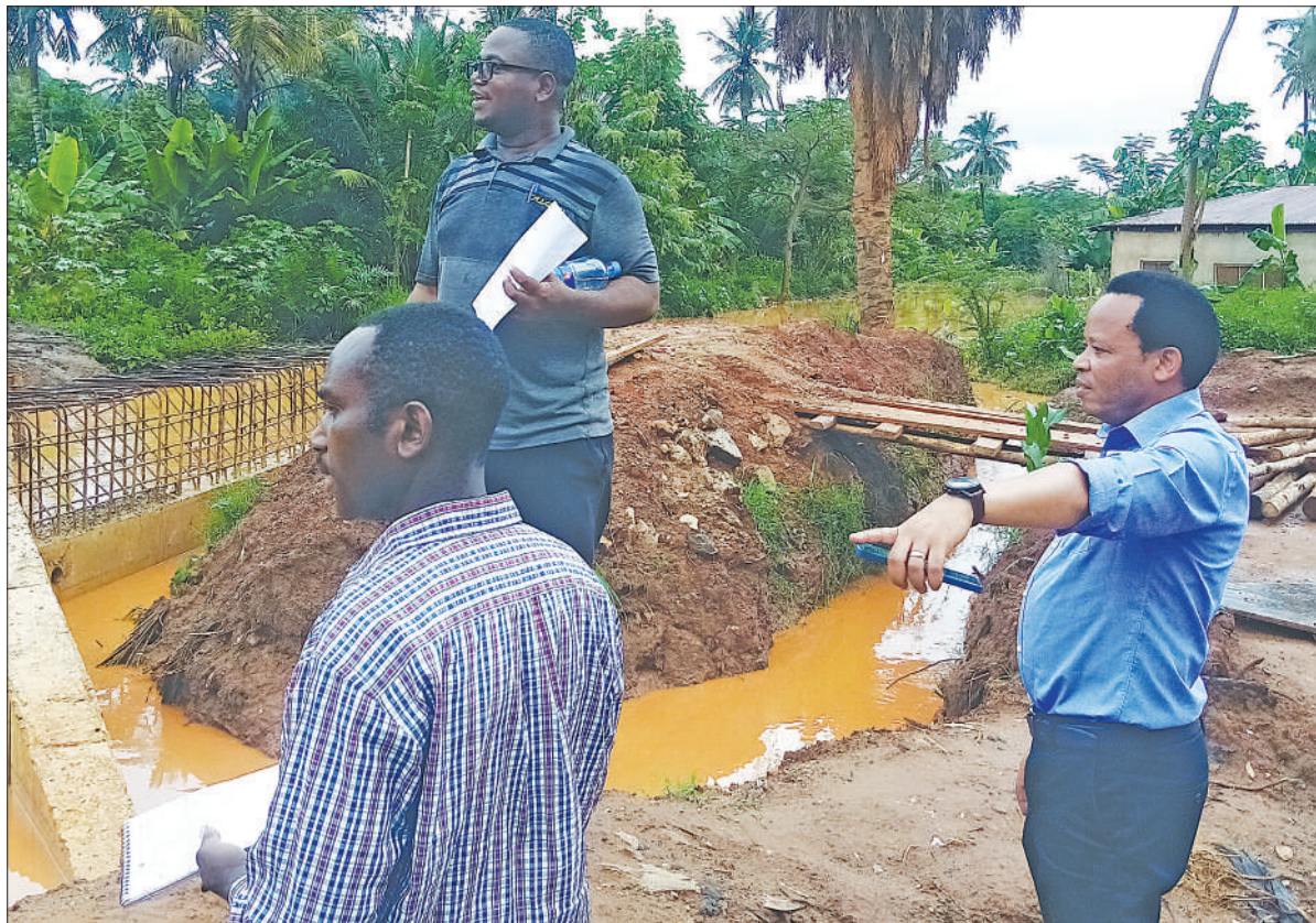
Muheza district administrative secretary Mohamed Mfaki (R) assesses progress in the execution of the Amtico Bridge construction project. The work has been put on hold for several days now owing to the ongoing rains. Photo: Correspondent Steven William
