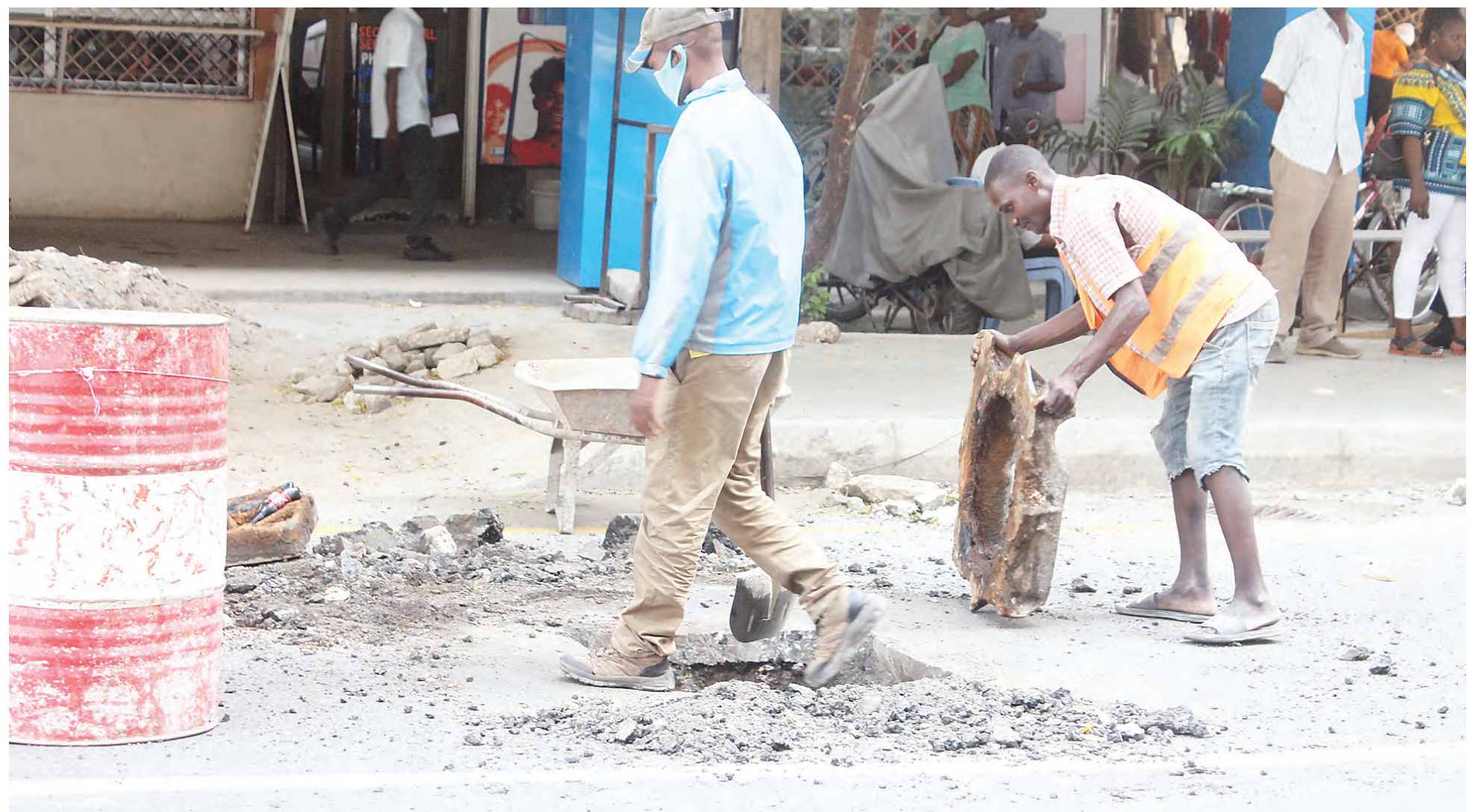
A drainage system along downtown Dar es Salaam's Samora Avenue undergoes repair earlier this week. Photo: Correspondent Jumanne Juma
