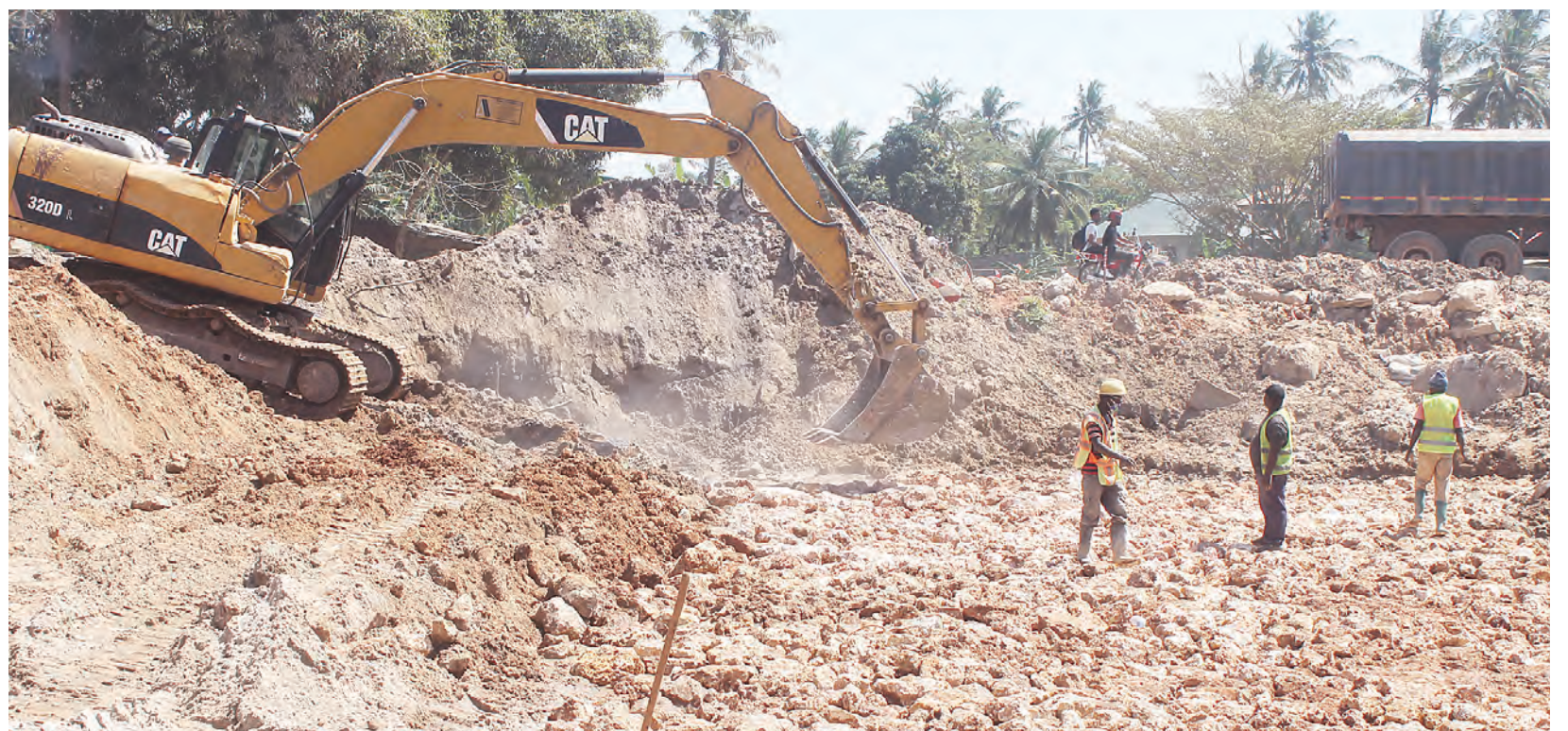
Preparations for the construction of Mzingo River Bridge in Dar es Salaam's Kitunda suburb well under way, as captured by Correspondent Jumanne Juma's roving camera yesterday. Photo:
