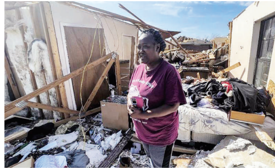
A woman stands inside her destroyed house in the aftermath of a tornado in Rolling Fork, Mississippi, on Sunday. (PHOTO / AFP)
