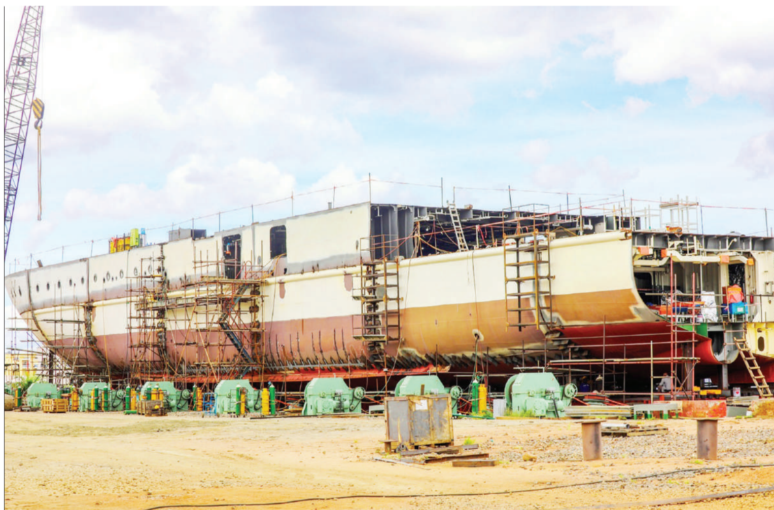
MV Mwanza christened 'Hapa Kazi tu' which is being rehabilitated by Ges Entec firm based in South Korea is now 74 per cent complete. The motor vessel will be completed next year. Works and Transport minister Dr Leonard Chamuriho (not pictured) inspected ongoing work progress on Tuesday. Photo: Guardian Correspondent
