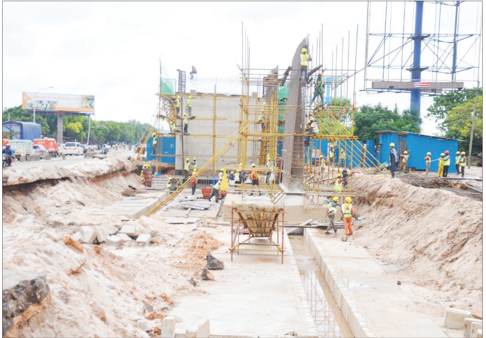
Chang'ombe flyover construction at the junction of Nyerere /Kawawa road in Dar es Salaam is going on under Chinese contractors to ease traffic jam as captured yesterday. Photo: Correspondent Jumanne Juma
