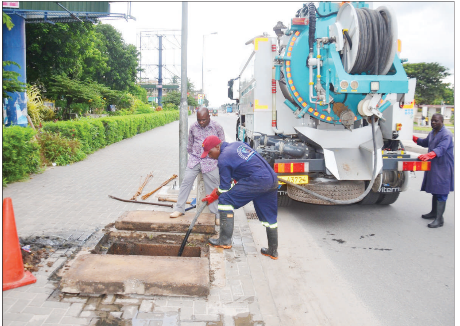
Dar es Salaam Water and Sanitation Authority workers unblock a sewage drain along Morogoro in Dar es Salaam on Tuesday. Photo: Correspondent Jumanne Juma
