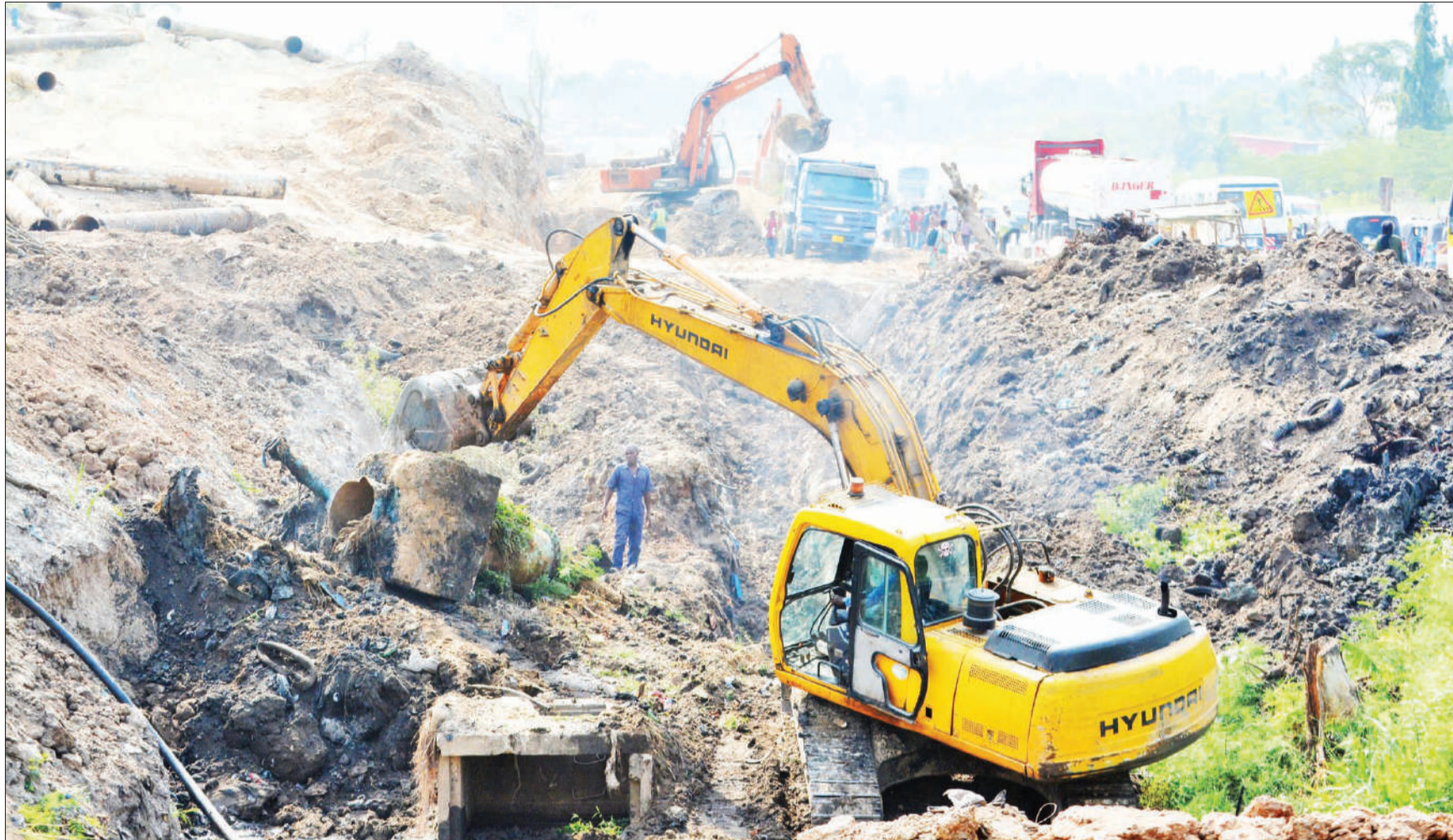
Expansion of the Morogoro Road stretch from Dar es Salaam's Kimara Mwisho suburb to Kibaha in Coast Region under way at Mbezi Mwisho in Dar es Salaam, as witnessed yesterday by Correspondent Emmanuel Mwamkinga of Turdaco.
