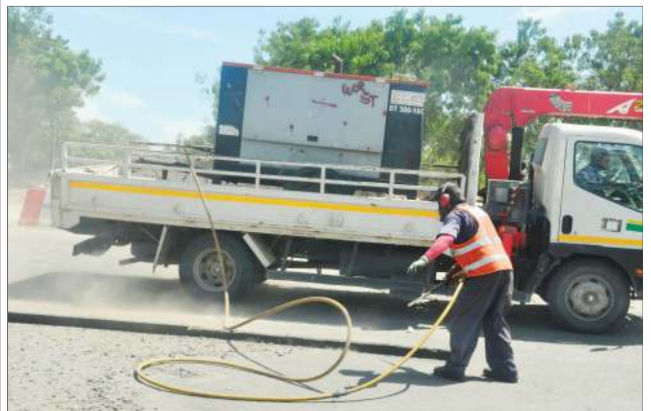
An Estim construction firm worker busy 'laying the ground' for the expansion of Morogoro Road into a six-lane dual carriageway from Dar es Salaam's Kimara suburb to Kibaha in Coast Region, as found at Kimara Temboni yesterday. Photo: John Badi
