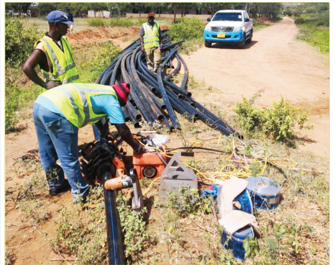
Dar es Salaam Water and Sanitation technicians laying water supply and sewerage pipe lines along the Same-Mwanga-Korogwe water project yesterday. Photo: Guardian Correspondent
